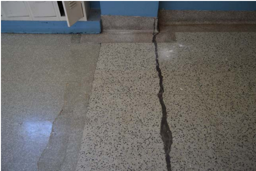
Fig. 144 Detail of upper-floor corridor where terrazzo floor in wing meets terrazzo floor in 1928 building
