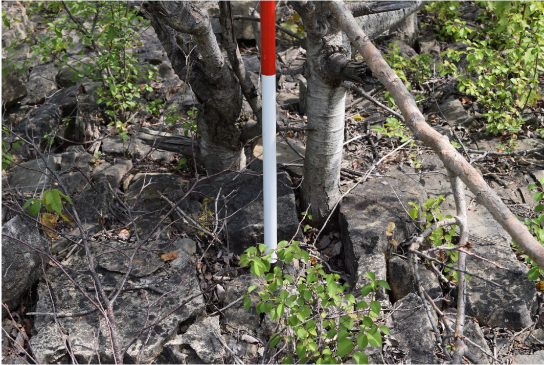
Figure 71: Root action dislodging stones of the coursed rubble lining of Barton Reservoir.
