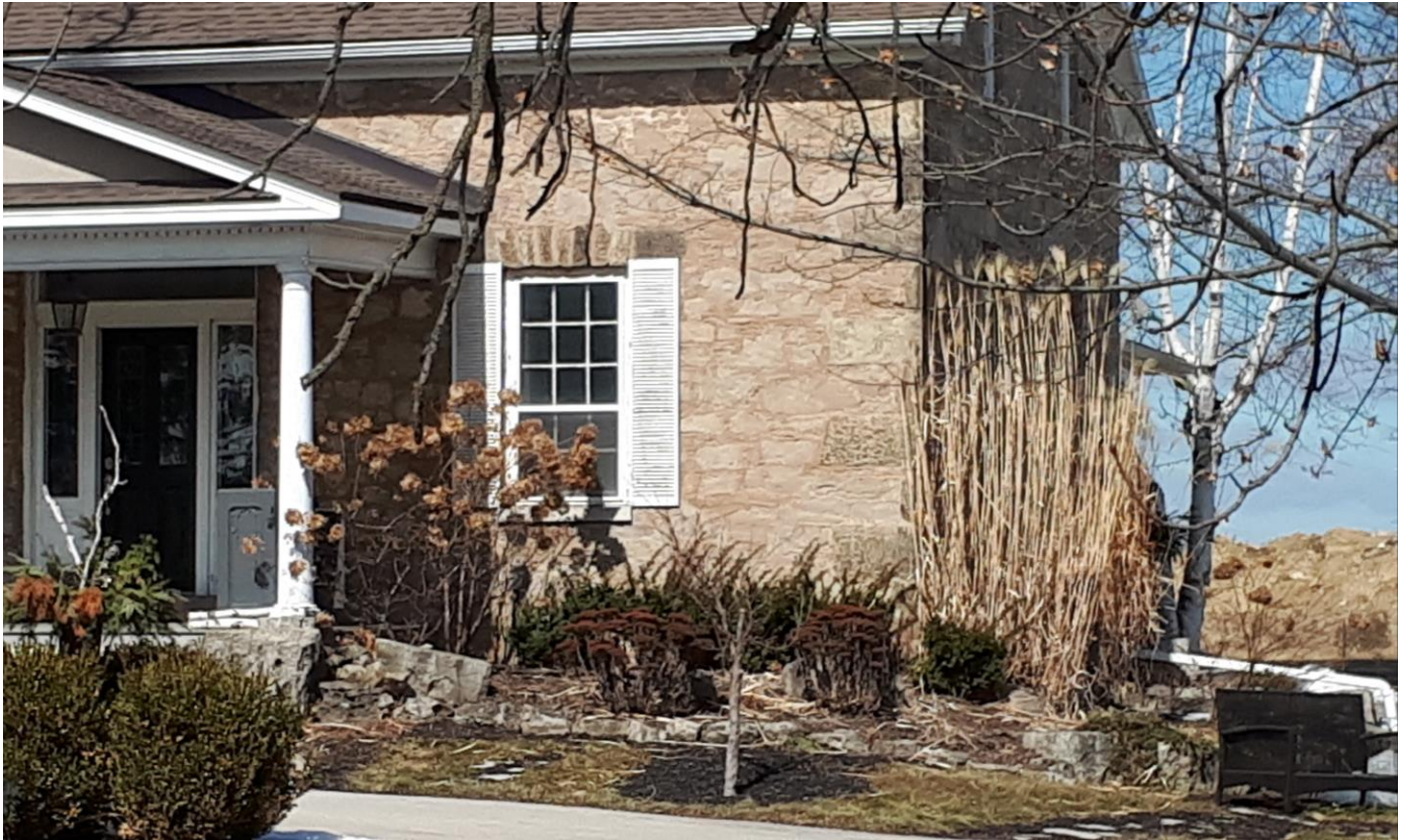
Figure 5: A closer image of the Lampman House's limestone masonry, comprising walls of rubble or fieldstone and cut sandstone quoin blocks (Parsons, 2018).
