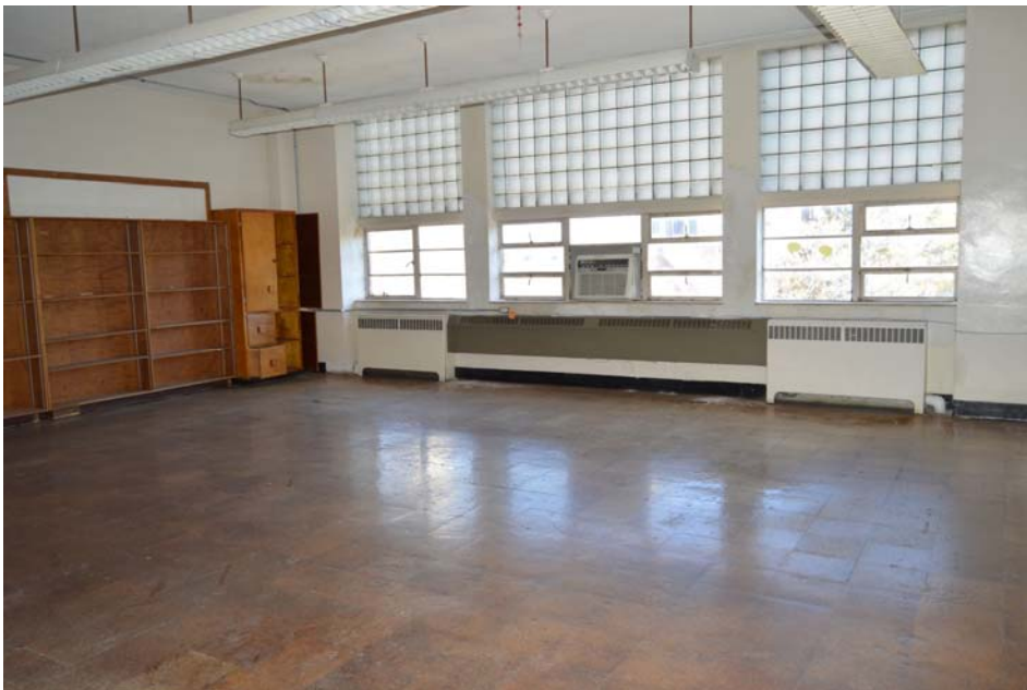
Fig. 146 Typical upper-floor classroom. Note cork floor and tripartite window with fixed glass block uppers and operable clear glass lowers.
