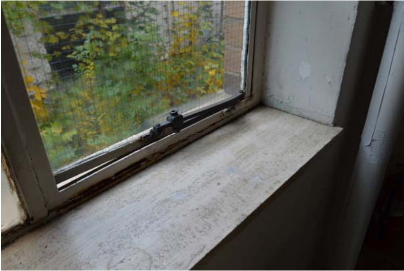
Fig. 135 Detail of window in ground-floor lobby. Note bronze hardware for the operable sash as well as the travertine marble sill.
