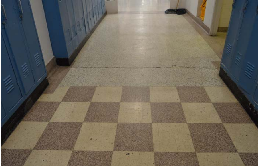
Fig. 141 Detail showing where wing's ground-floor corridor in grey and brownish terrazzo meets 1928 building's checkerboard terrazzo
