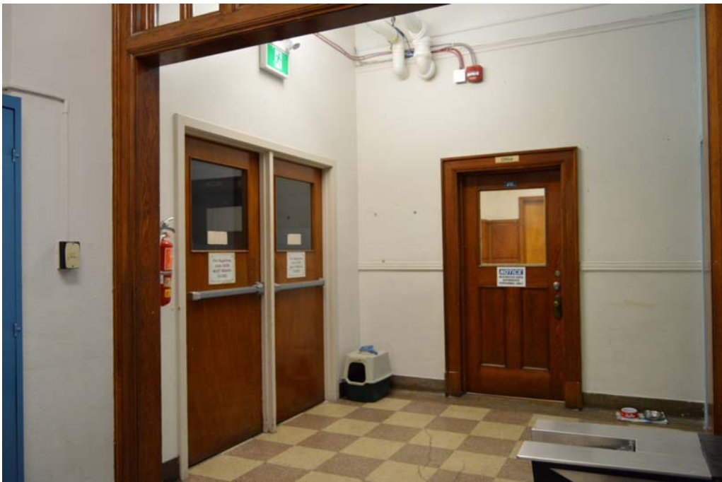
Fig. 79 Place on ground floor where the east-west corridor meets the north-south corridor. Note fire separation partition and fire doors to the left of the frame, door to the administration office, wood-framed transom light over the north-south corridor opening, and terrazzo floor in a checkerboard pattern.
