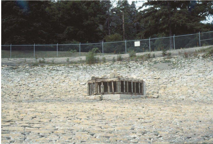
Figure 34: Circa 1970s photograph of the east main pipe and housing (courtesy HMST).
