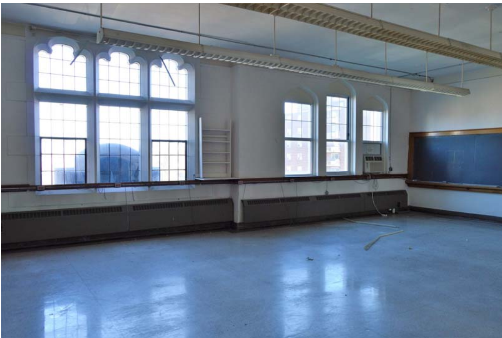
Fig. 110 Room 28 tripartite windows. Note that the sash on the left is original and the sash on the right is a replacement.
