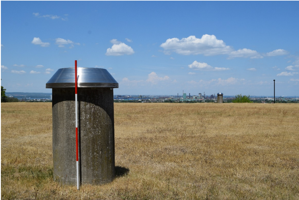
Figure 61: The concrete vent pipes on the north and south boundaries of the reservoir.
