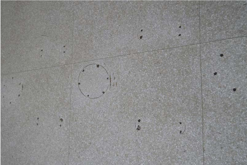
Fig. 101 Room 26 terrazzo floor marred with holes
