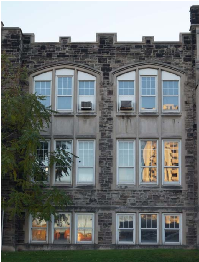
Fig. 45 Windowed bays to either side of the entrance bay. Note this view shows the bays east of the entrance bay.
