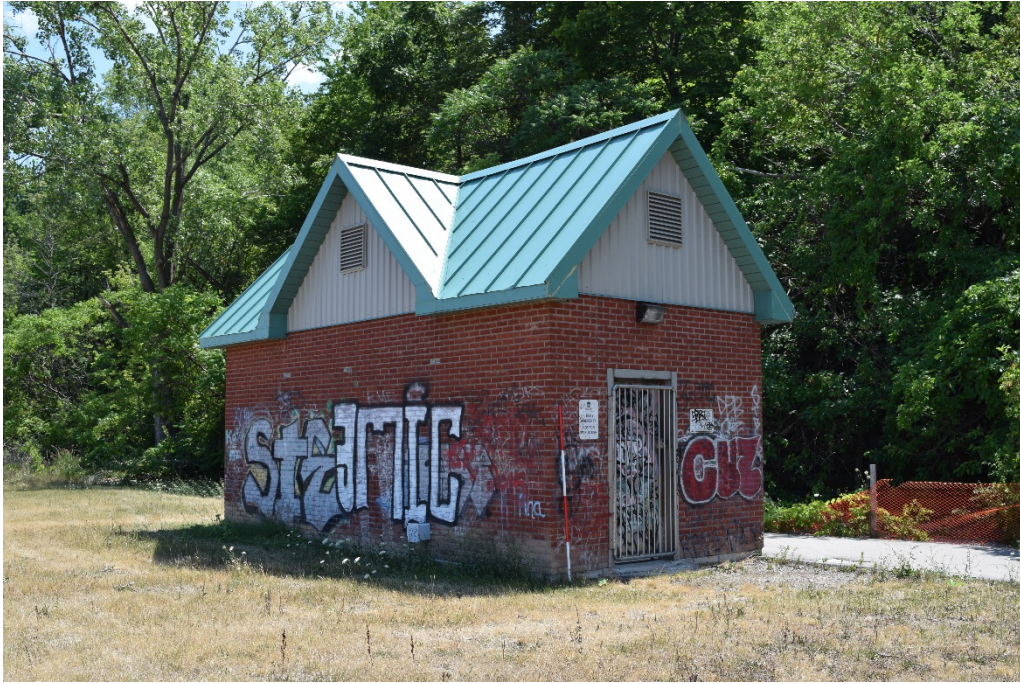
Figure 62: View facing southeast of the brick building in the south-centre portion of the reservoir.
