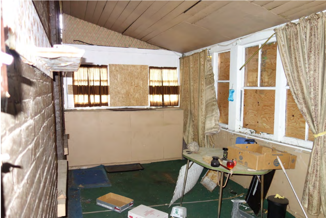
Porch – east end – the floor has collapsed at this end
