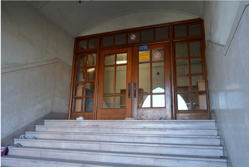
Fig. 35 View as seen inside the entry porch, looking up the marble staircase to the doorway into the school's front vestibule
