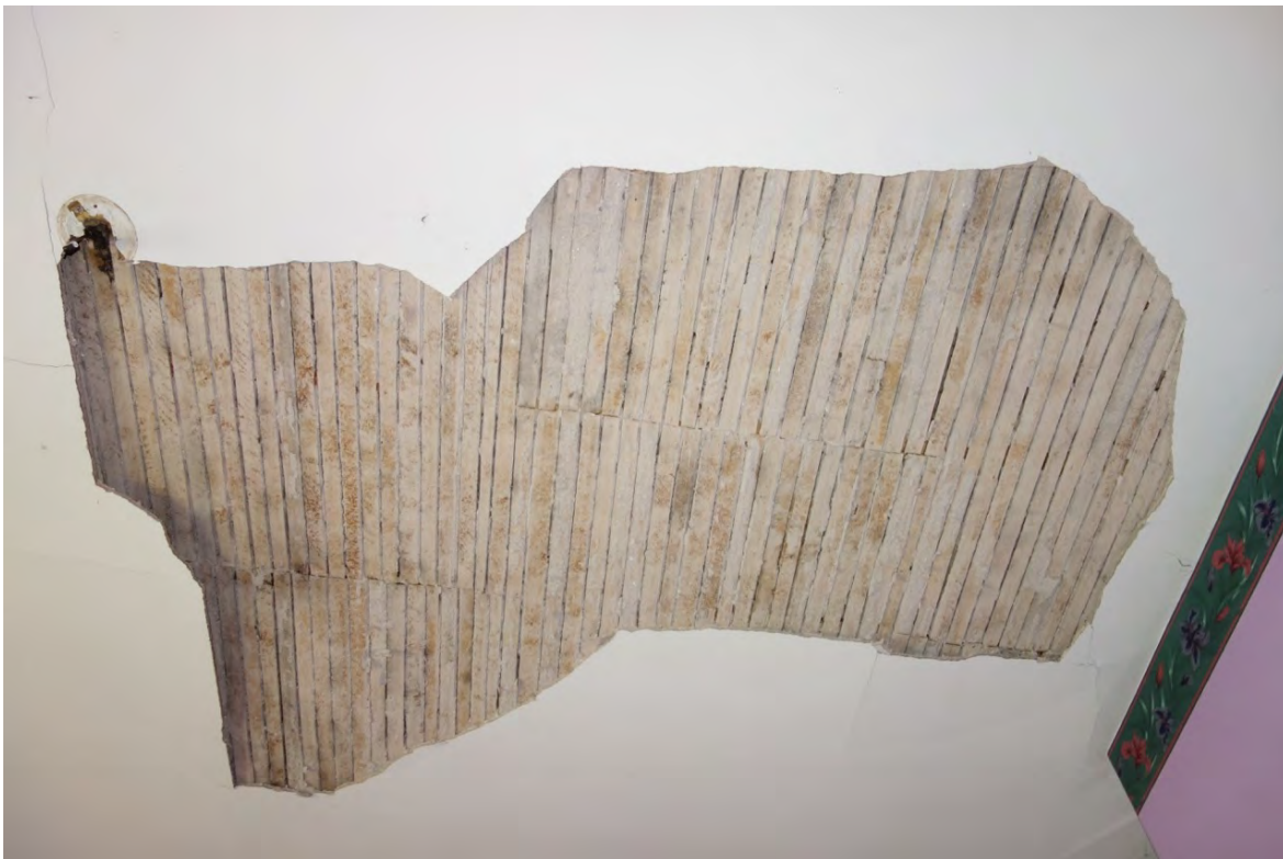
West parlour – ceiling plaster damage
