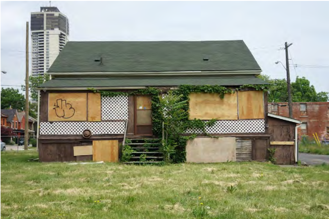
122 Augusta Street – vacant and boarded up
