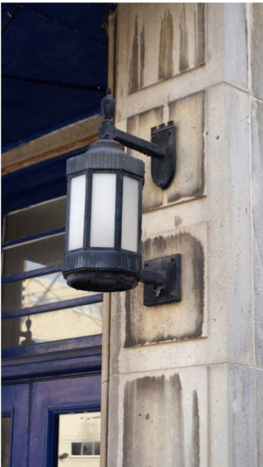
Fig. 74 Wall-mounted lamp at wing's entrance
