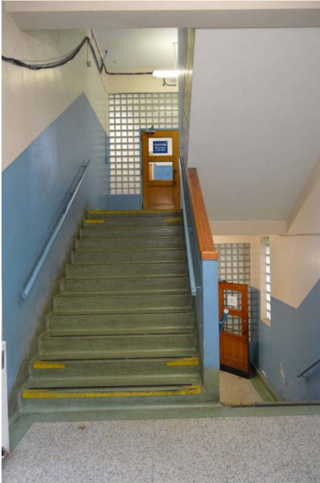
Fig. 131 Stairwell inside entry to wing, looking up to the ground floor and down to the basement
