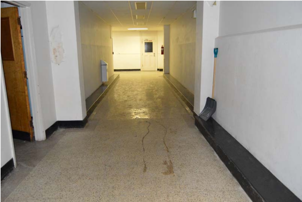
Fig. 153 North-south corridor in wing's basement, looking from the cafeteria northward to the east-west basement corridor of the 1928 building
