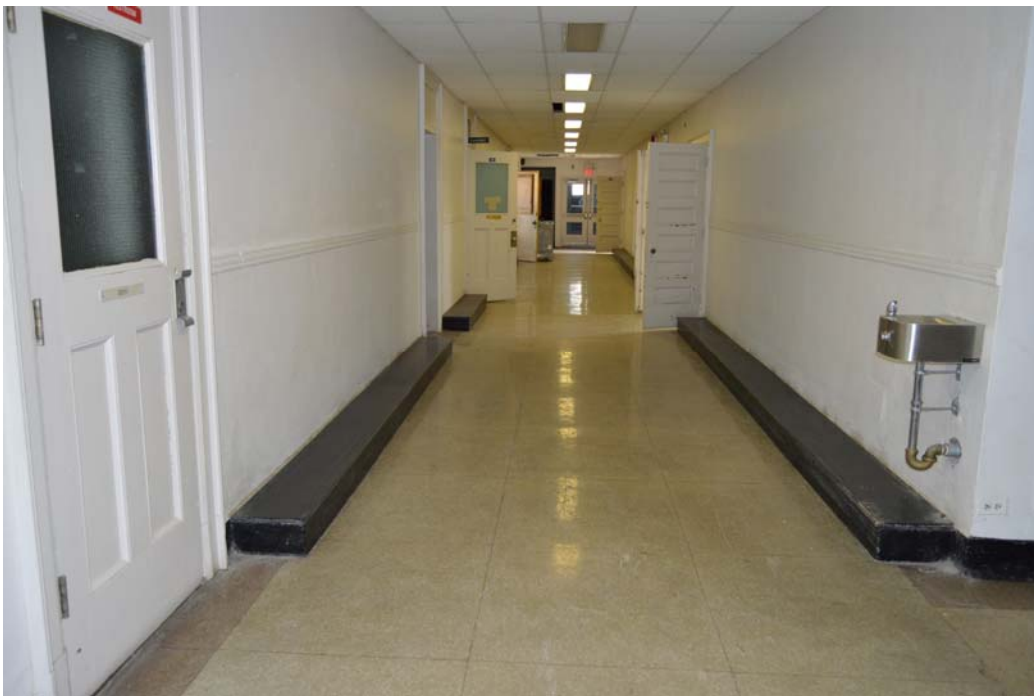
Fig. 118 East-west corridor in basement, looking east. Note grey terrazzo floor with darker terrazzo border.
