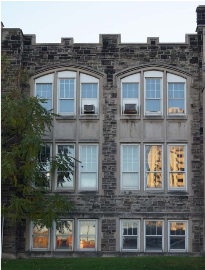
Fig. 45 Windowed bays to either side of the entrance bay. Note this view shows the bays east of the entrance bay.
