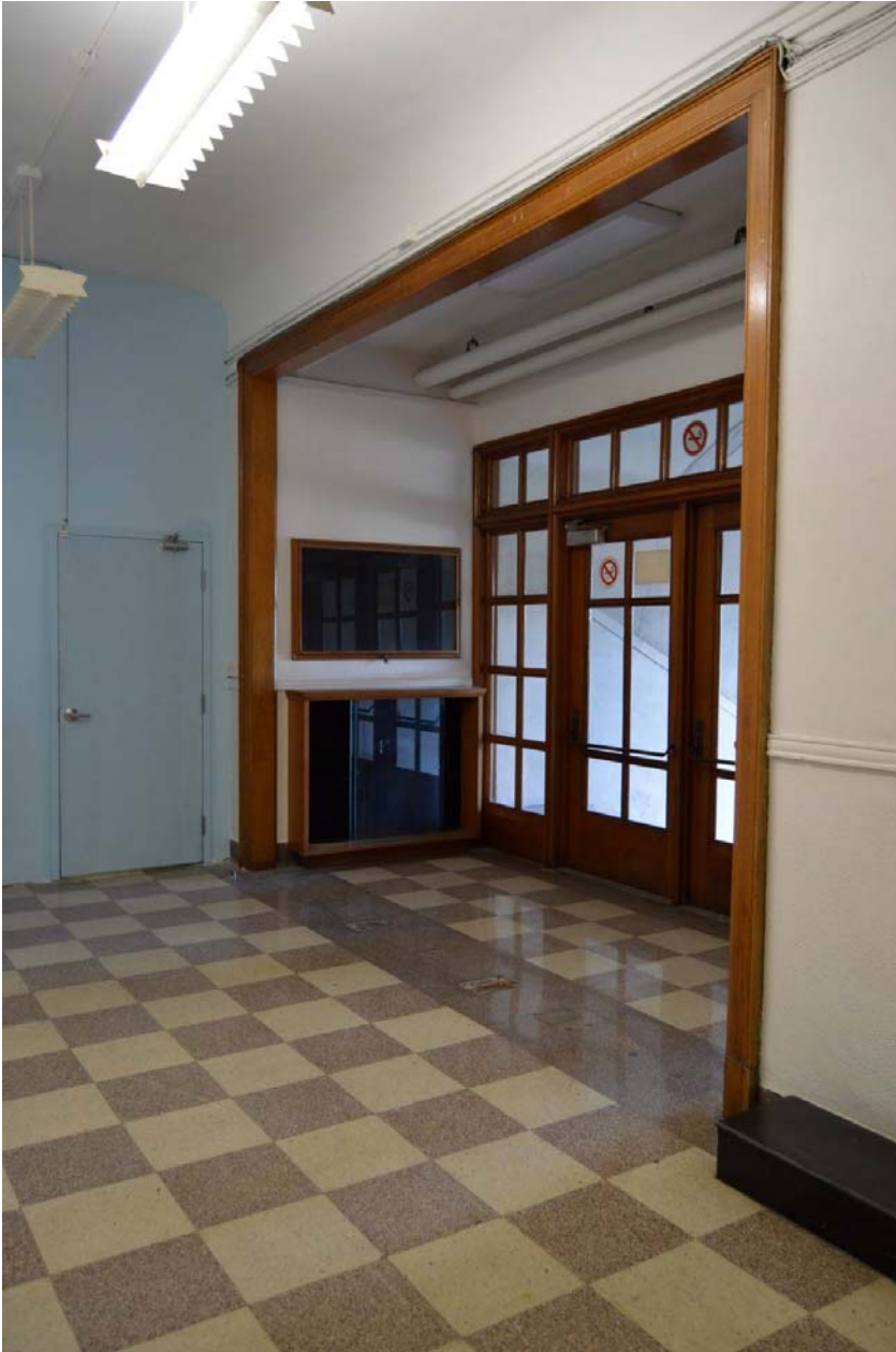
Fig. 86 Front entrance vestibule with fire separation partition on left of frame. Note holes in floor where the vestibule doors once stood.
