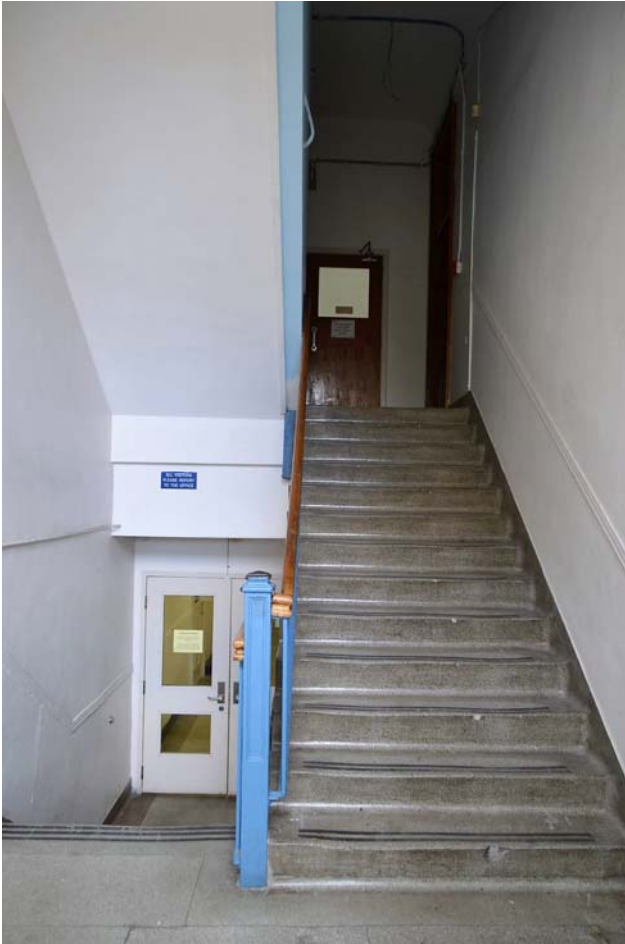
Fig. 77 West entrance staircase immediately past west entrance vestibule, looking up to the ground floor and down to the basement. Note the metal newel post, metal balusters, wood handrail and terrazzo risers and treads – all dating to the 1928 construction.
