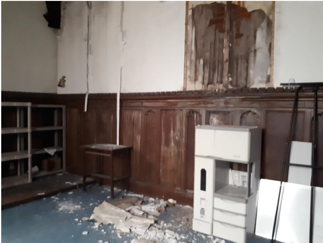
Water damage in Memorial addition, May 31, 2018
