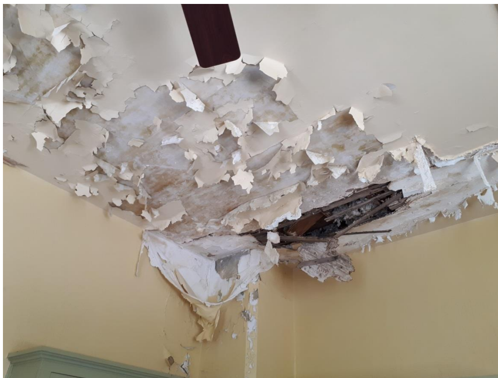
Water damage in room above arched entrance on Holton Avenue South, May 31, 2018
