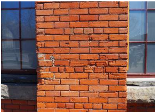
Figure 4.13 - Damage to original brick, possibly from vehicles entering/exiting garage.
