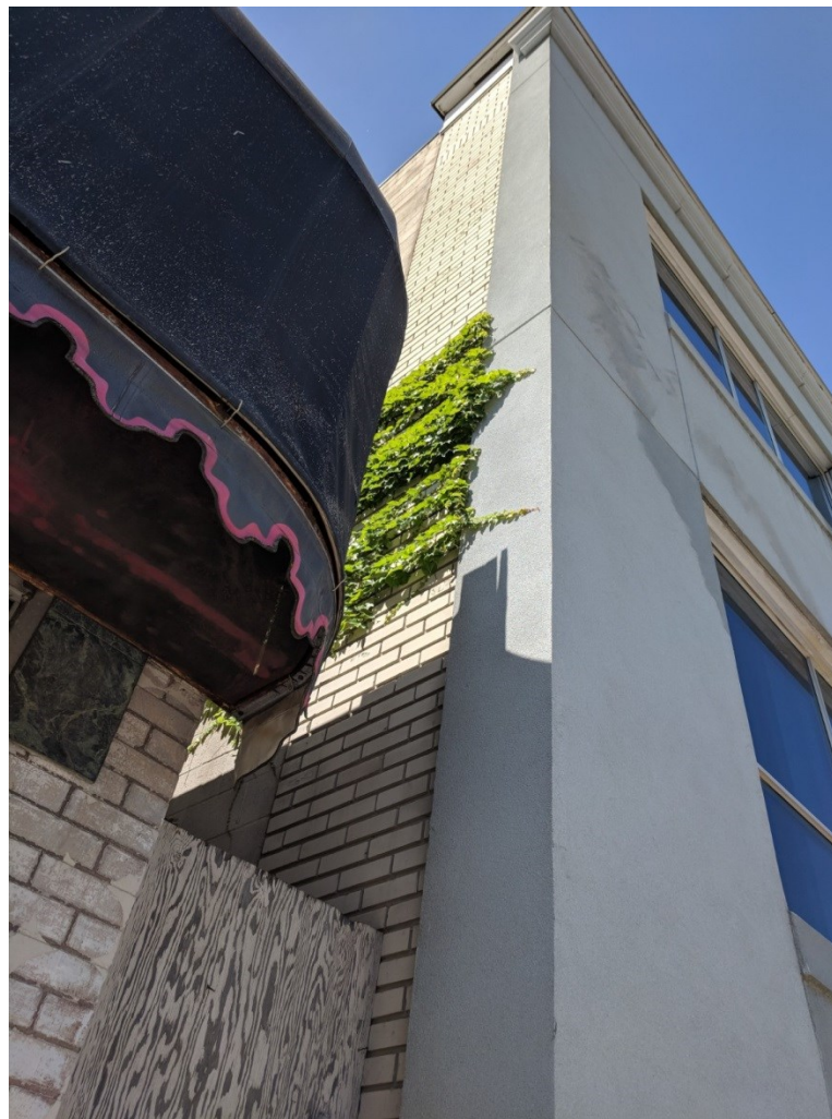
Image 6: Photograph of the yellow brick exposed on the east side of the building (2018).
