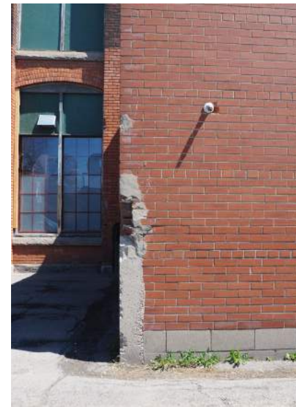
Figure 4.10 Brick Detail Damaged brick and poured concrete corner of garage
