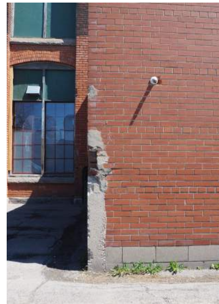
Figure 4.10 Brick Detail Damaged brick and poured concrete corner of garage
