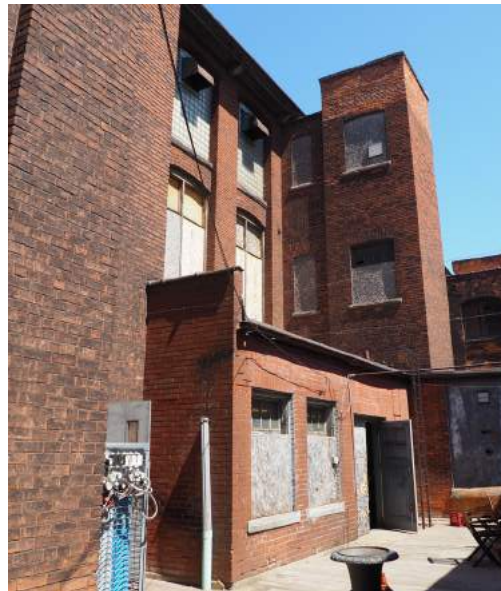
Figure 4.9 Courtyard View to south elevation from courtyard. All original openings with plywood and glass block infill with aluminum picture windows.
