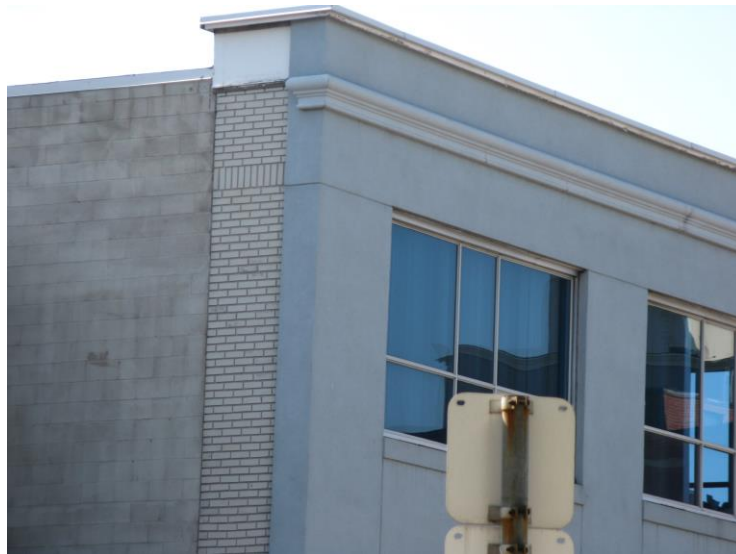
Image 4: Photograph of the yellow brick exposed on the east side of the building (2011).
