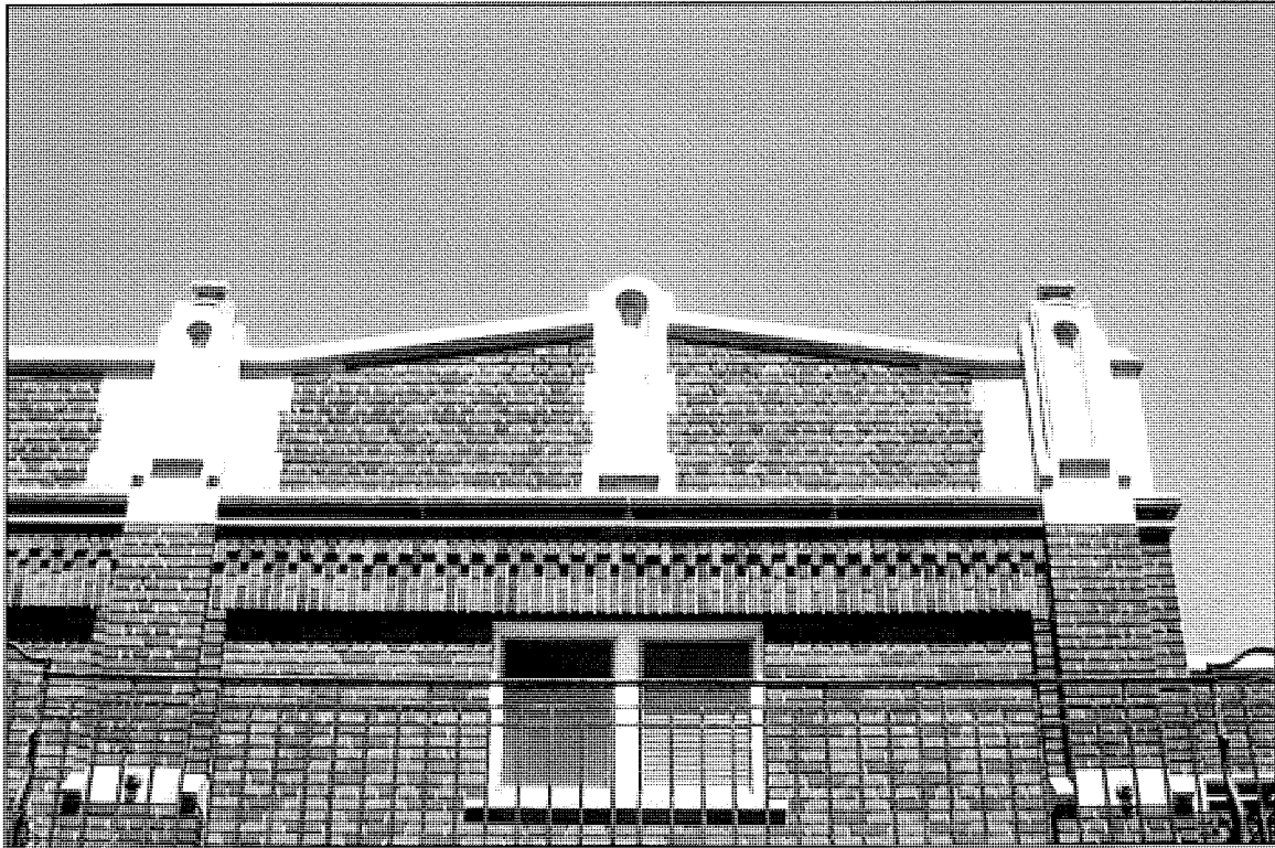
A pedimented parapet with concrete detailing highlights the end bays of the southwest wall.
