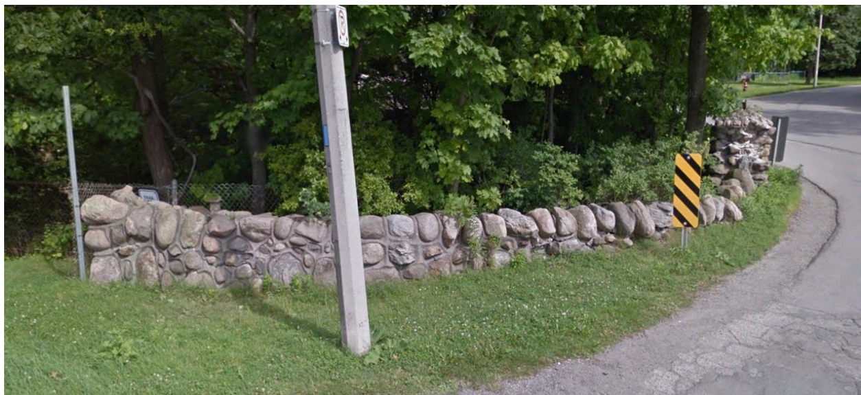
Figure 18: An image of the stone wall and pillars located between Sanatorium Road and the brow's edge (Google Street View, 2015).
