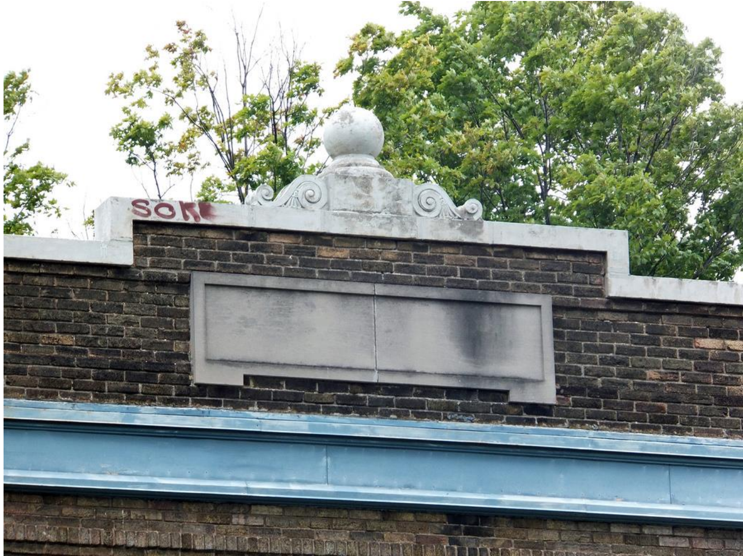
Decorative finial feature and inset stone atop the building's modest parapet . The simple blue frieze board is visible below. (Flickr, 2014).
