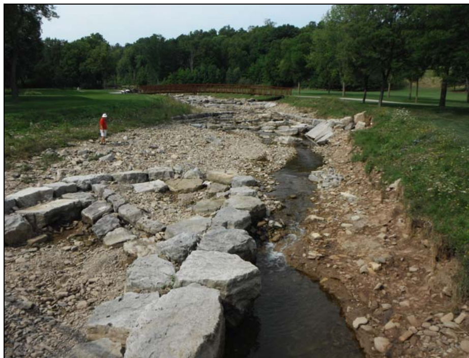
Figure 5. Red Hill Creek post-flood event on August 9 th , 2012 showing extensive scouring of the channel bank and loss of vegetation in King's Forest Golf Course.
