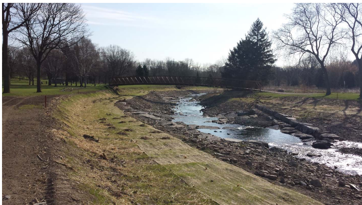
Figure 2.4.3 2015 channel works through King's Forest Golf course which shows increased golf cart bridge spans, floodplain benches and modified in-stream structures.
