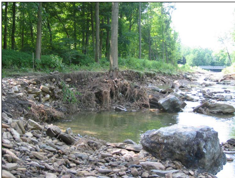
Figure 4. Extensive erosion of the creek channel and embankment following the flood on July 29th, 2009. King's Forest between transects 2 and 3.
