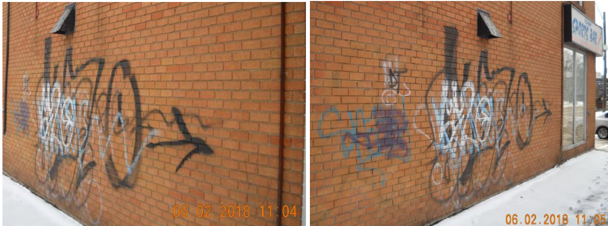
Before photos taken on February 6th 2018 at commercial property on Queenston Road.
