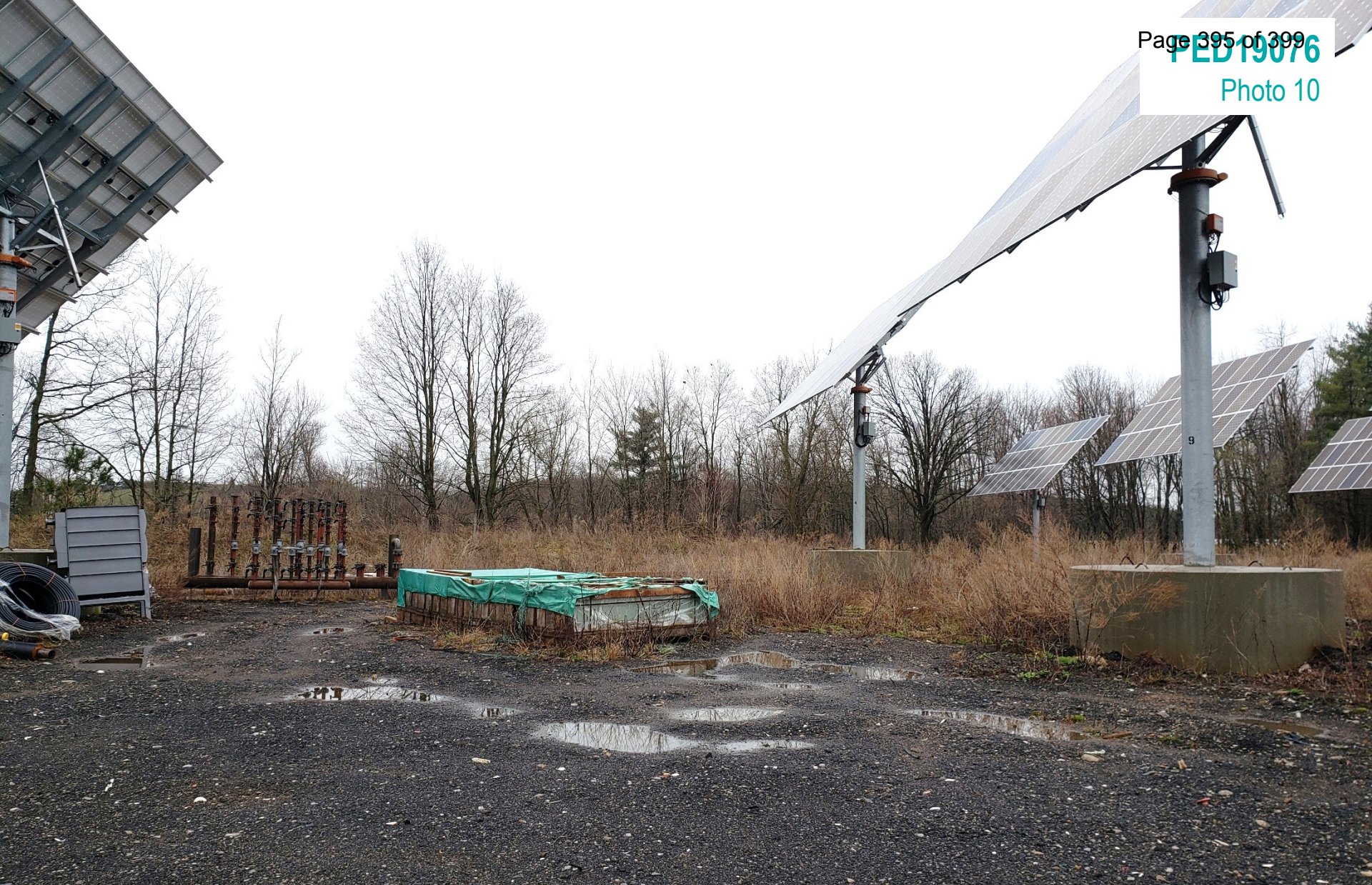
Solar Panels to the south
