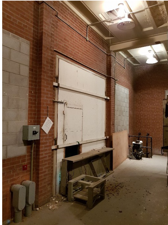
Figure 70: South wall entrance and blind windows of the 1955 Extension facing southwest. The ladder to the basement is in the far corner.
