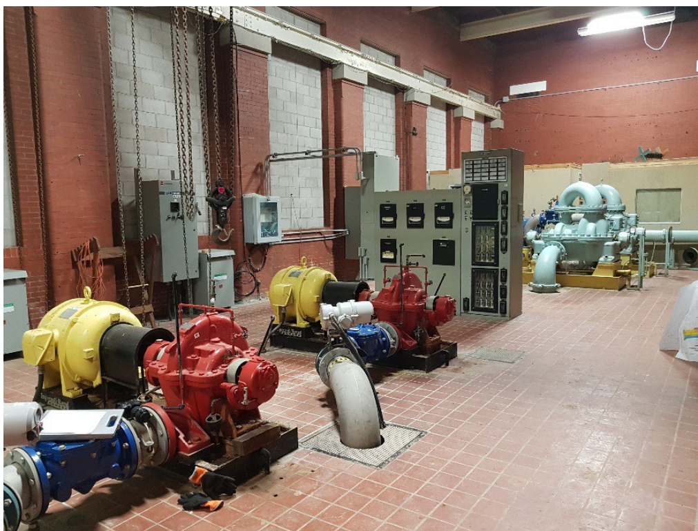
Figure 52: Mountain Level Pump Trains, High Lift Pump Trains, and Control Panel on the north portion of the floor.
