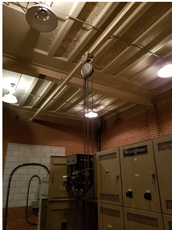
Figure 71: Fire proof ceiling with elliptical lights, and Columbus McKinnon Cyclone 1/2-ton beam trolley with hanging chain hoist.
