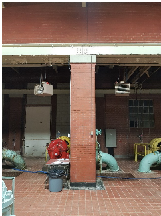
Figure 63: Chamfered and corbelled pillar or column supporting the 1929-30 breach into the 1912-13 Block, as seen facing south from inside the 1912-13 Block.
