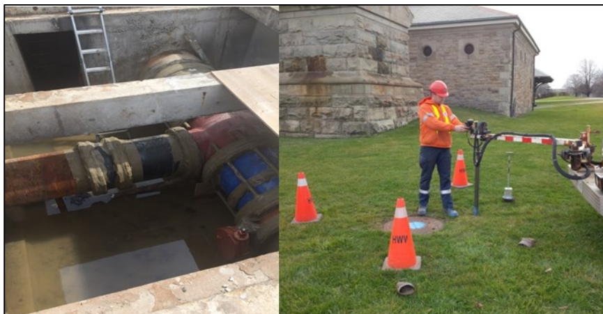
Water valves preventative maintenance
