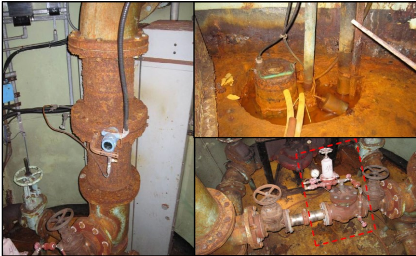
Main st w/Whitney Ave. water pumping station (1968) Replacement value - $4.9M
