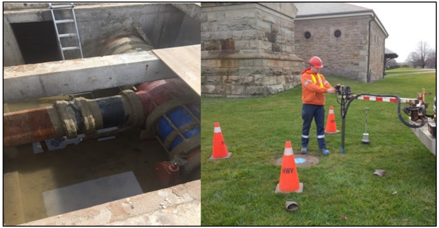
Water valves preventative maintenance
