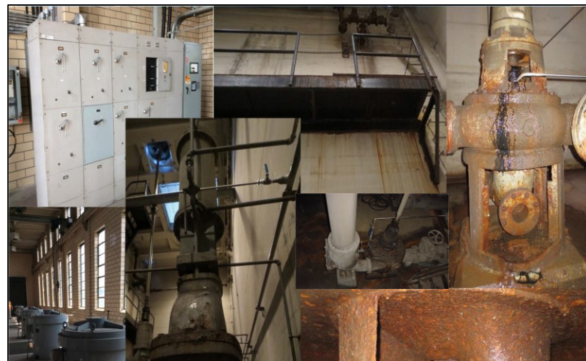
Parkdale Ave. wastewater pump station (1955) Rehabilitation value - $6.08M
