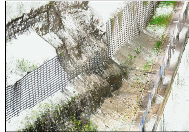
Escarpment Bin Wall damage
