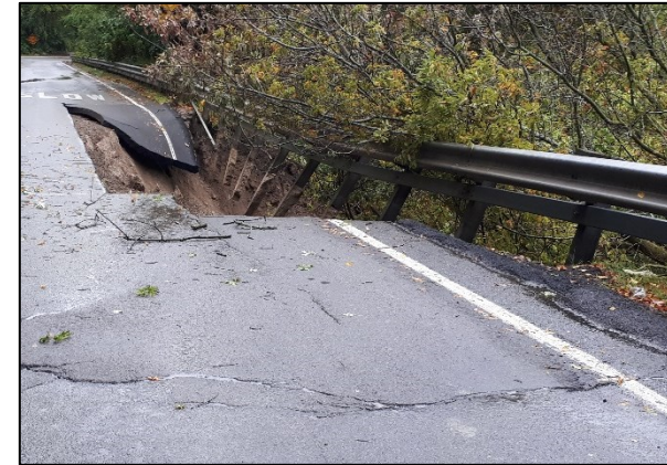
Hwy 8 Dundas Escarpment Failure
