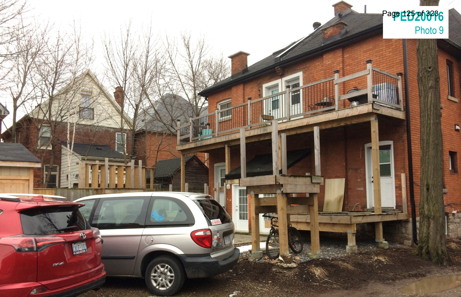
Rear of the subject property, as seen from the alleyway looking south east
