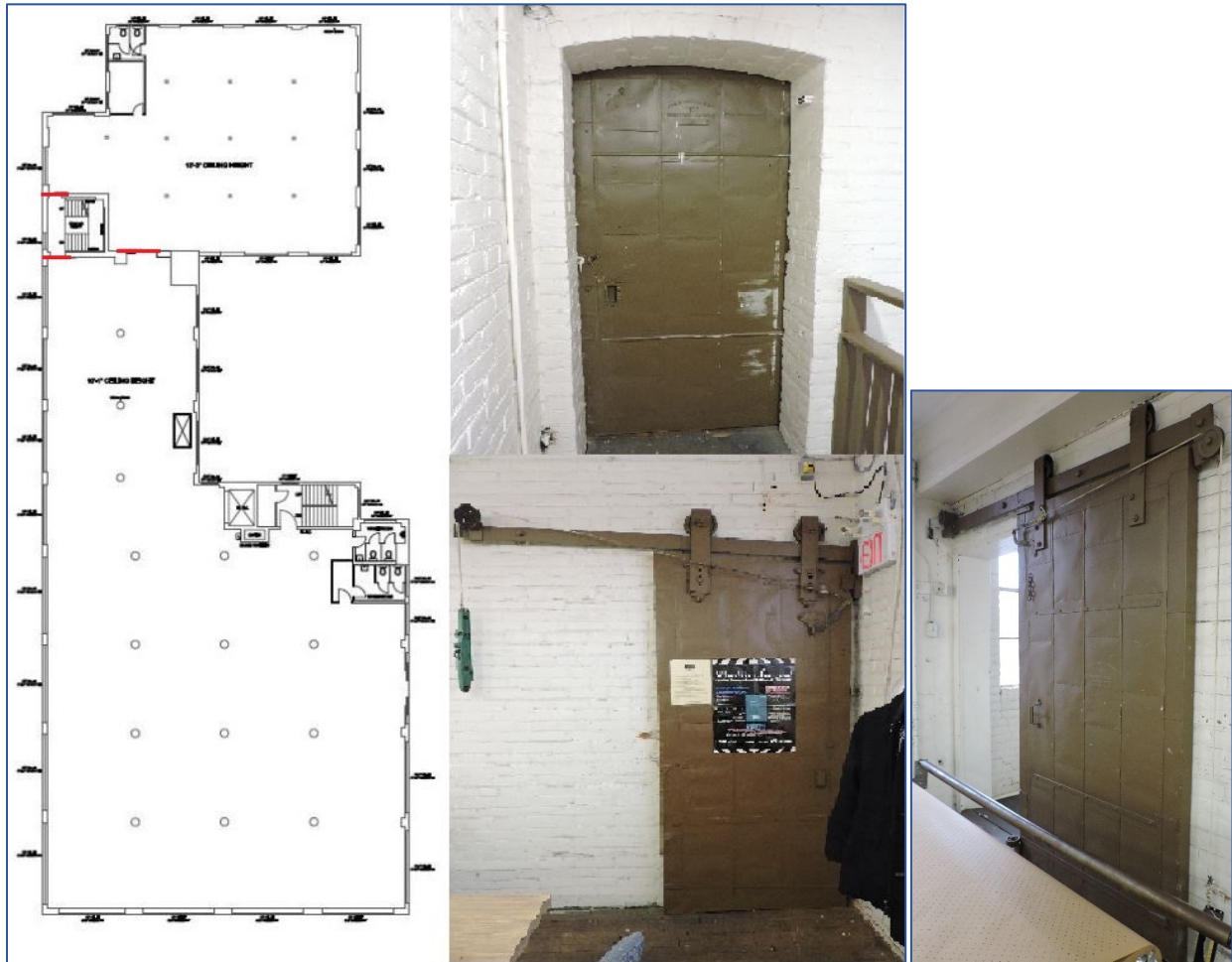
Figure 43: Second level plan with fire door locations marked in red. The two photos on the left show the single fire doors located in the stairwell. The photo on the right shows the large fire door which separated the two sections of building (ZH, 2018).
