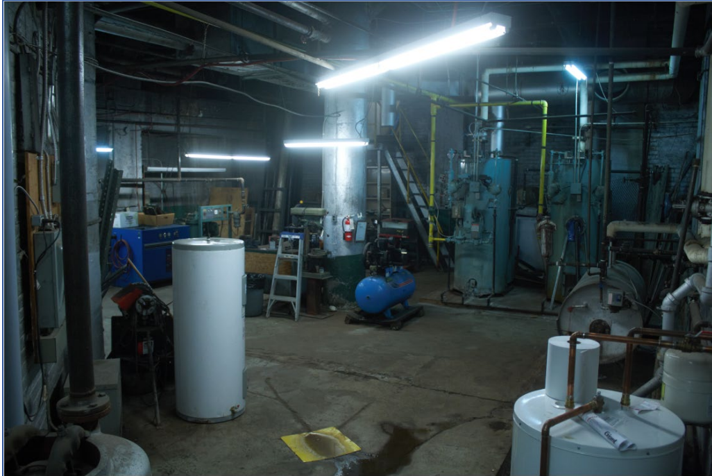
Figure 49: Boiler room (ZH, 2018).
