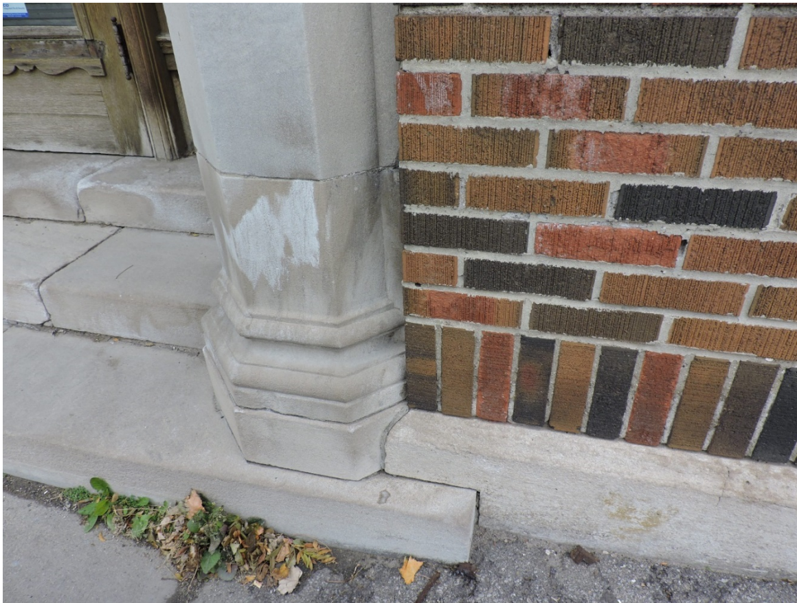
Figure 20 Front entrance, showing concrete steps, pillar base, brickwork, concrete foundation transition (AB, 2018).
