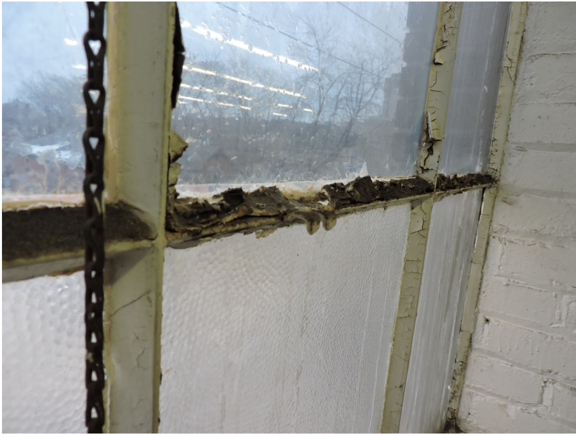
Figure 61 Interior window condition in west section (AB, 2018).
