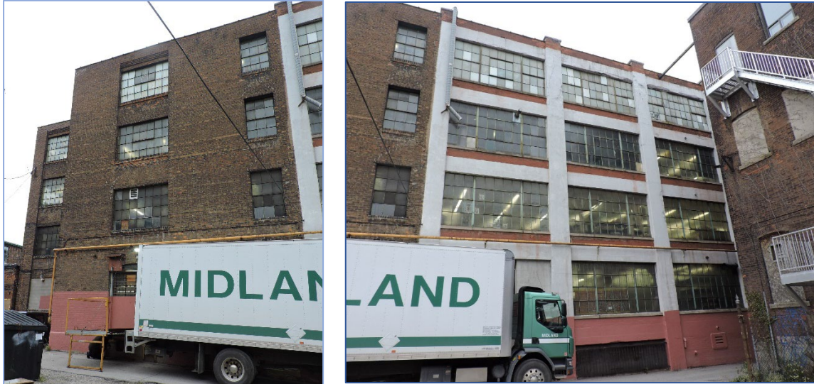
Figure 33: South elevation, showing where 1911 building on (left) meets c.1929 building (right). Note the 1929 building is covered in parking and painted (AB, 2018).
