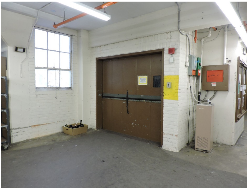
Figure 56: Fourth floor, elevator (AB, 2018).
