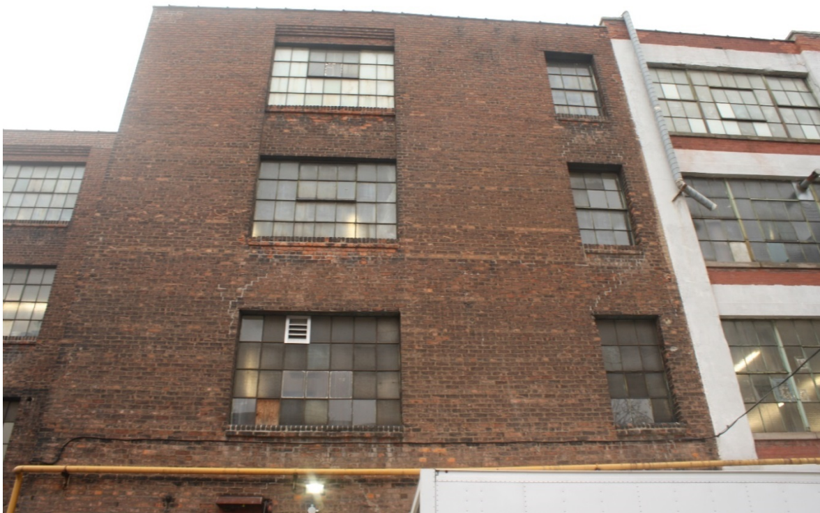
Figure 10 South side wall transition between east (right) and west (left) sections (ZH, 2018).
