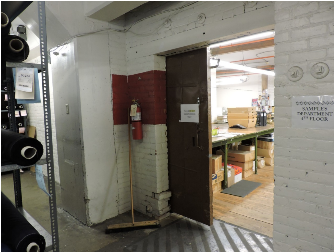
Figure 50 Fire door between east and west sections (AB, 2018).
