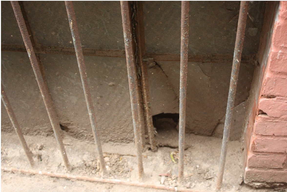
Figure 9 Deteriorating barred basement windows on south wall of the east section (ZH, 2018).
