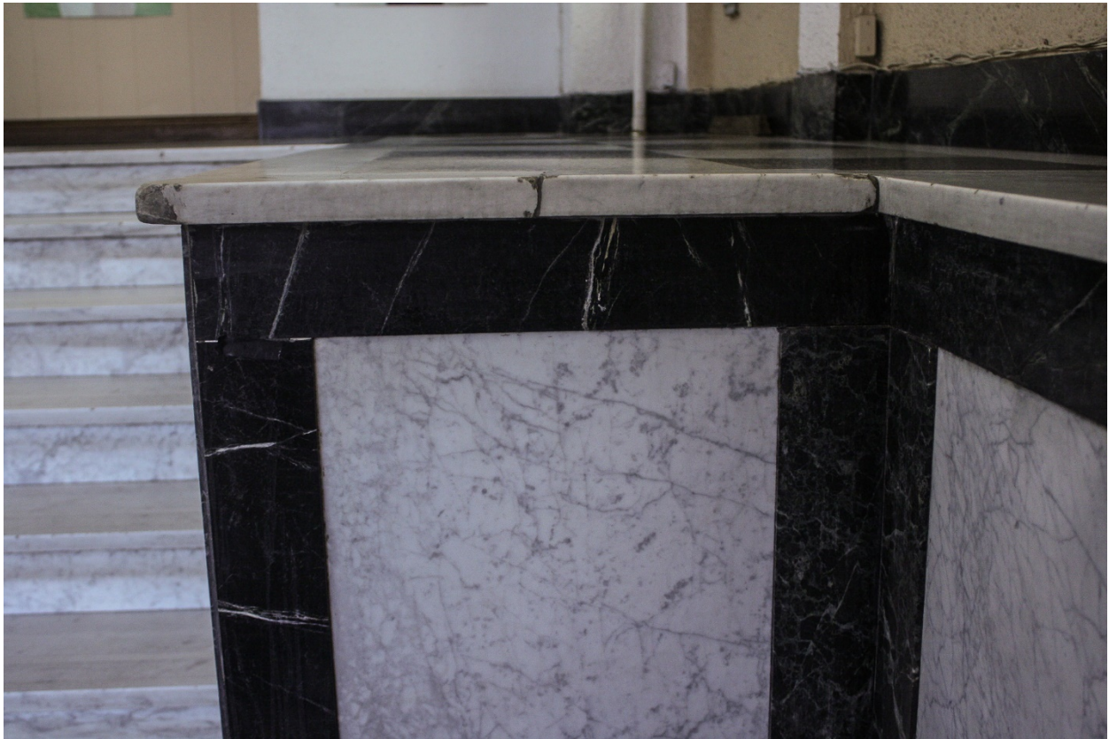
Figure 36 Foyer – showing black and white marble trim of split level beside staircase (ZH, 2018).
