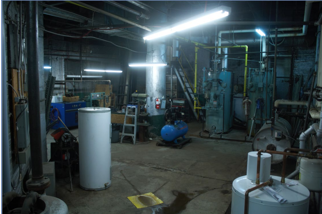
Figure 49: Boiler room (ZH, 2018).
