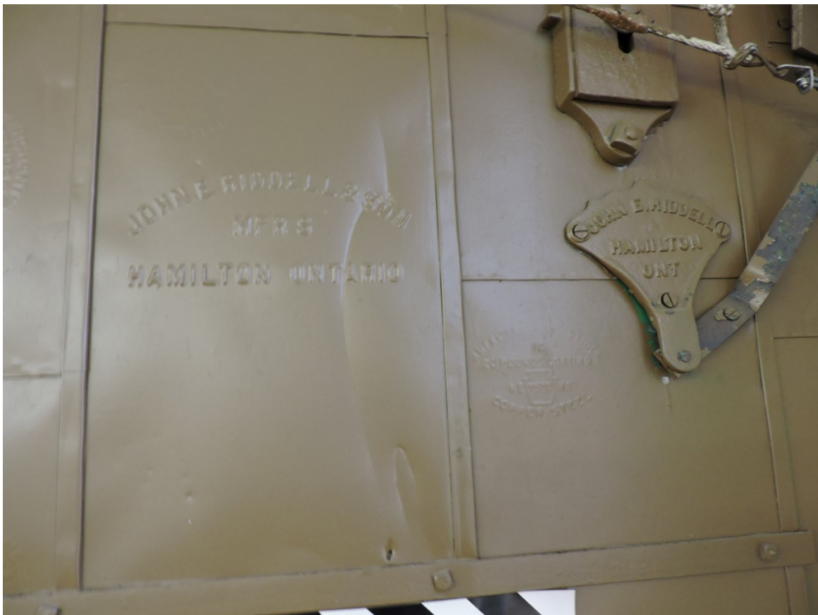
Figure 55 Fire door detail – John E Riddell and STM Manufacturers, Hamilton, ON (AB, 2018).
