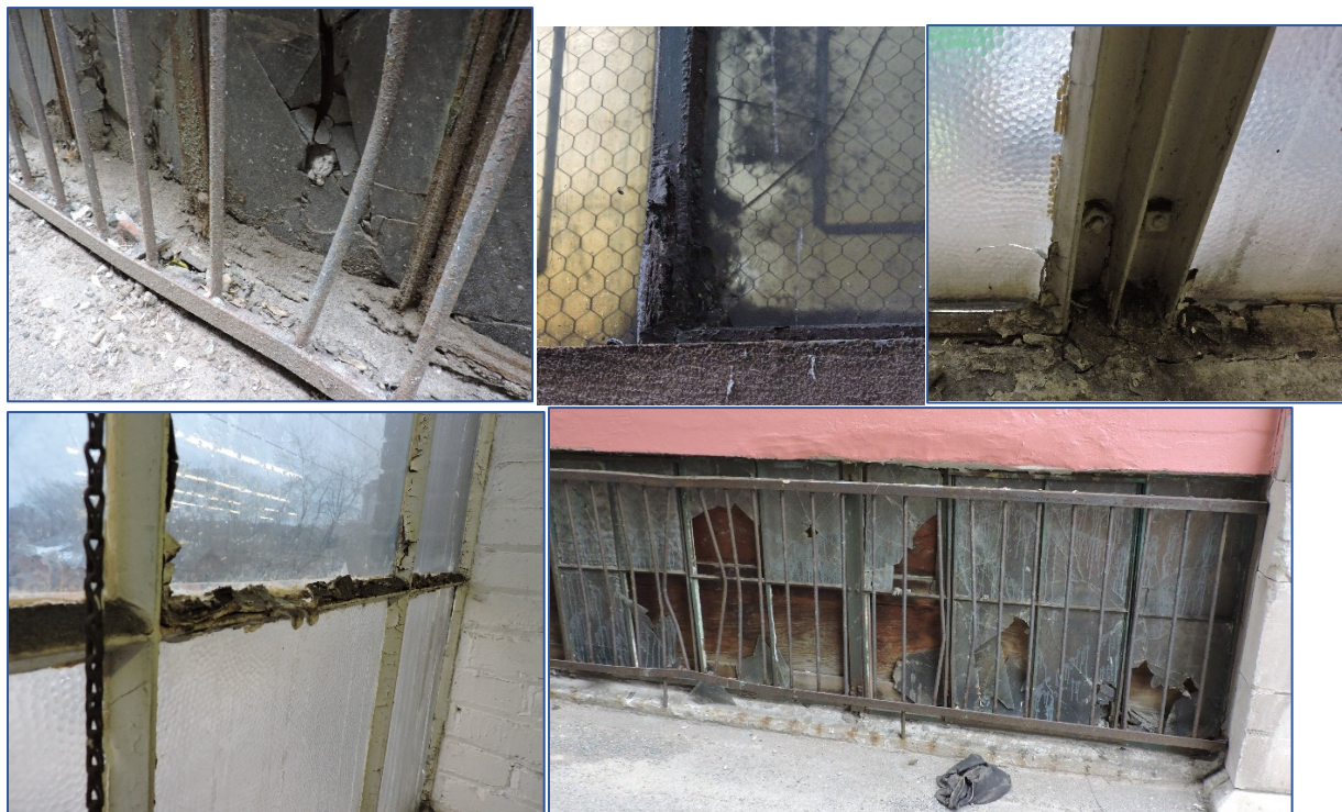
Figure 34: Examples of damaged or failing windows (AB, 2018).
