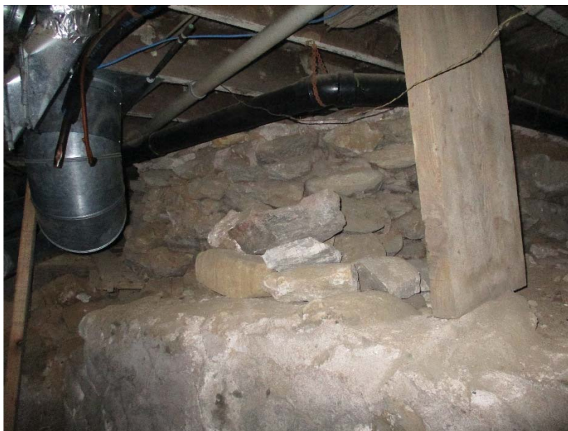
Later basement wall (foreground) supporting earlier shallow wall (background) Also note temporary prop under failing joist
