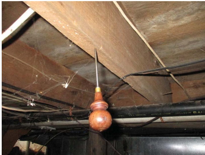
Deteriorated floor joist, awl inserted >2"
