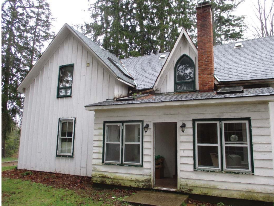
North side showing various roof issues
