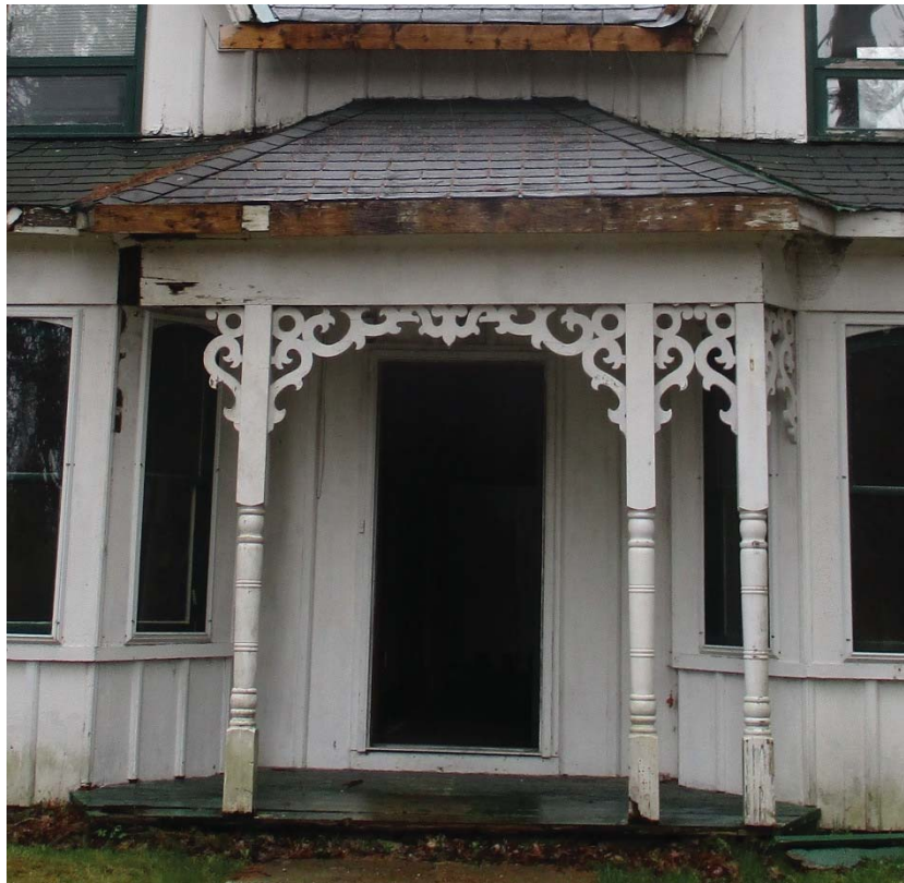
Porch with upside-down posts
