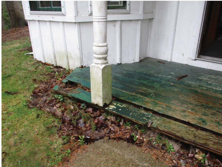
Front porch with rotting modern post and failing floor structure
