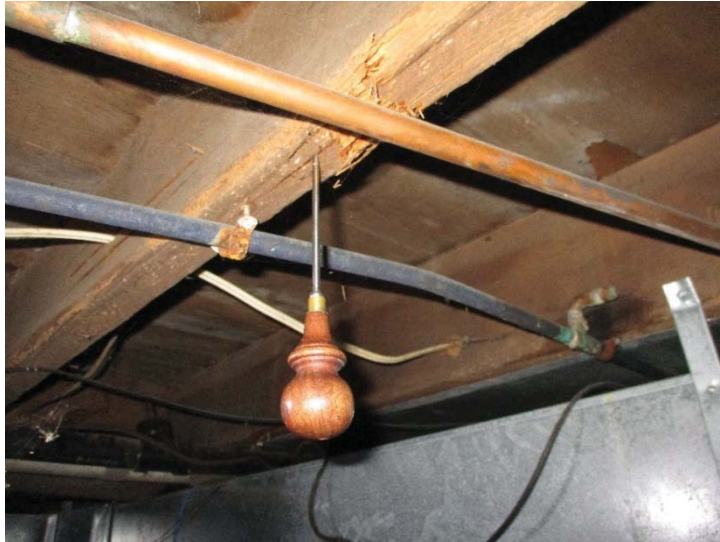
Deteriorated floor joist, awl inserted >2"
