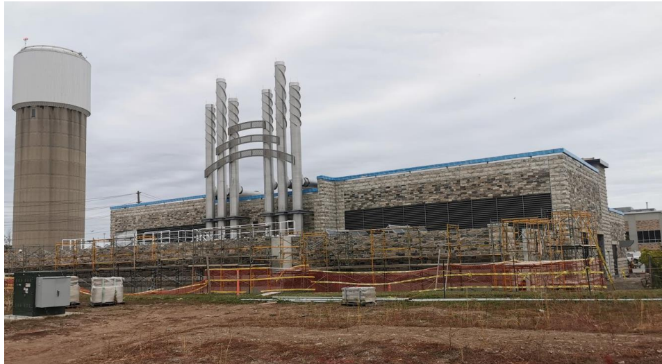
Figure 4: New Electrical Power Centre
