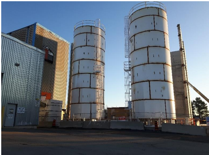
Figure 3: New Biosolids/Wet Sludge Storage Silos (2018)
