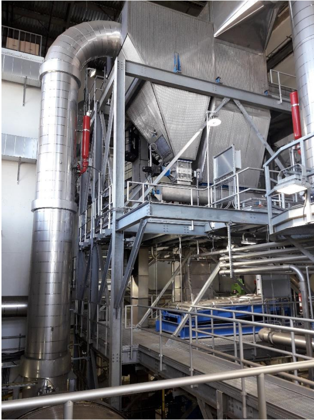
Figure 7: Facility Interior; Shaker Screen and Separator (2020)
