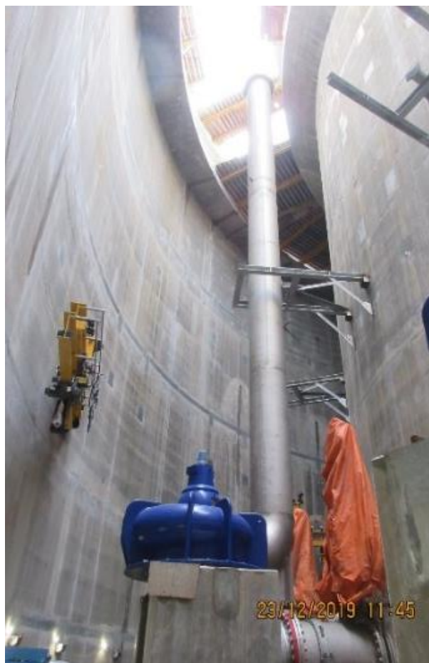
Figure 3: New Pump and Piping
