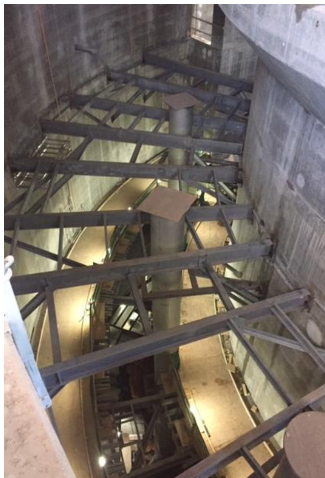
Figure 1: New Main Pumping View from Top of Dry Well
