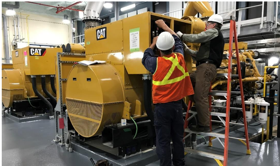
Figure 5: New 3 Mega-Watt Diesel Generator
