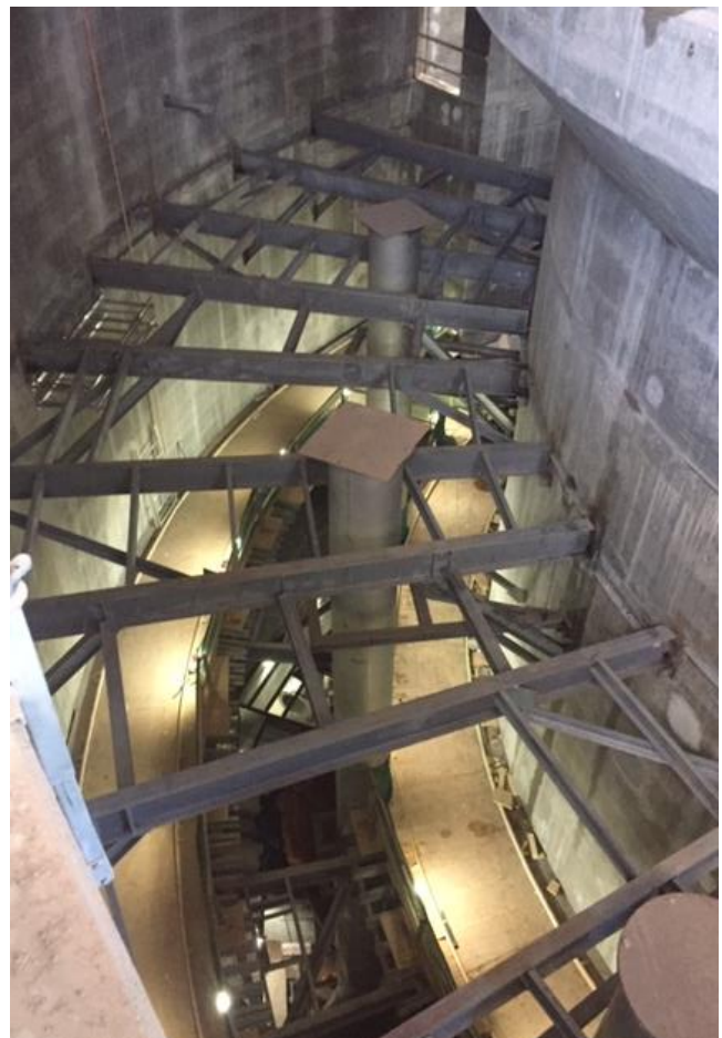
Figure 1: New Main Pumping View from Top of Dry Well
