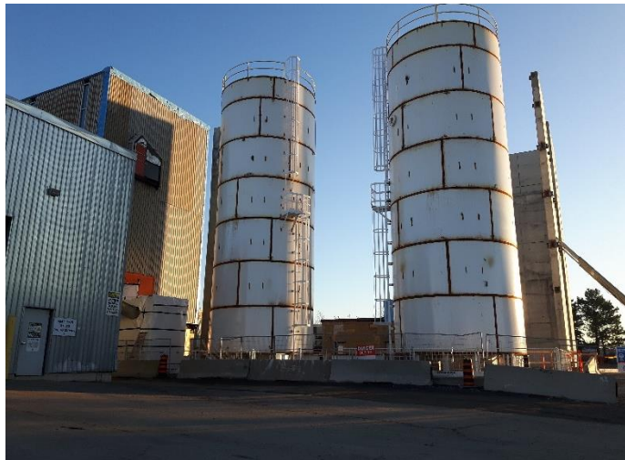
Figure 3: New Biosolids/Wet Sludge Storage Silos (2018)
