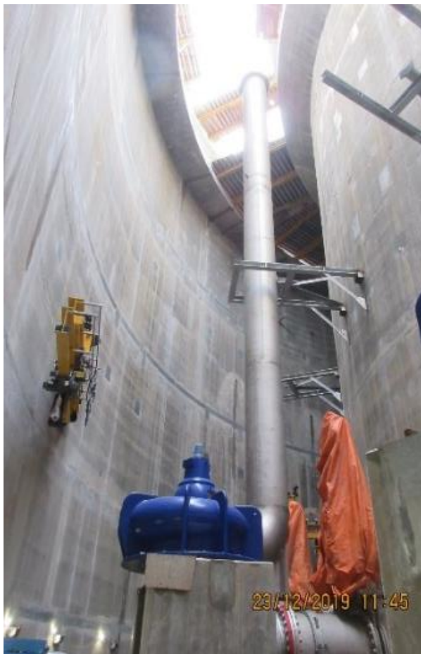
Figure 3: New Pump and Piping
