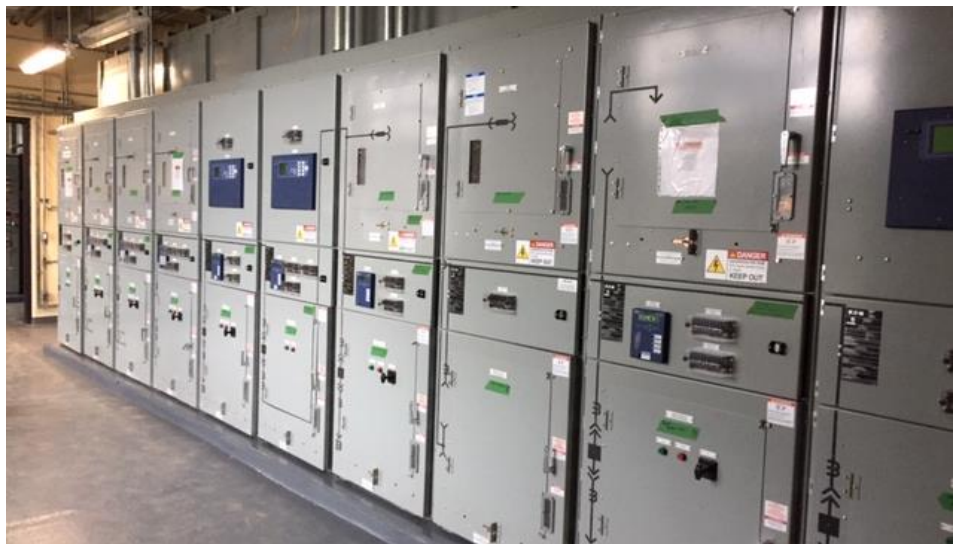
Figure 6: New Switchgear in Electrical Power Centre
