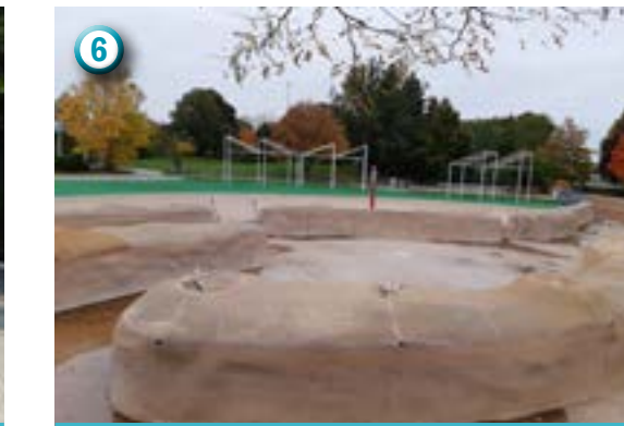
6 Exposed spray nozzle pipe poses a safety risk. Caulked joints are unsightly and collecting mold.
