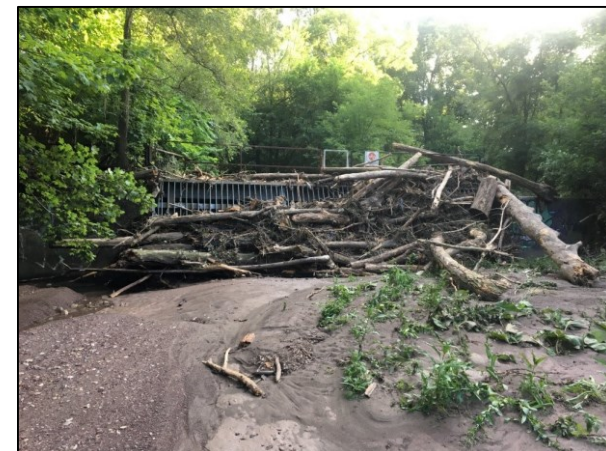
Chedoke SW inlet / outlet – near Chedoke golf course
