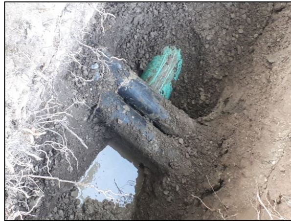
Sewer lateral damage – Markland St.
