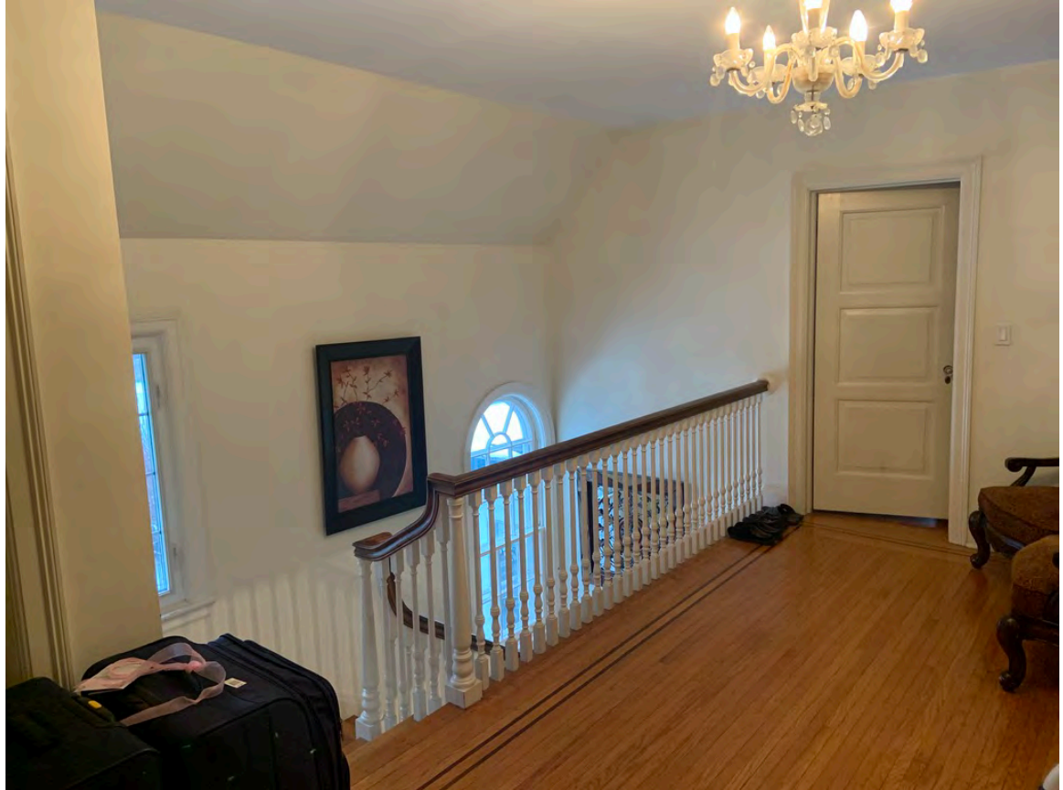
Second floor hall and sloping roof above the stairwell. The window heads are uncomfortably different and below eye level when standing on the second floor.
