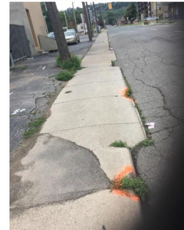
Uneven Surface Deflection 75
