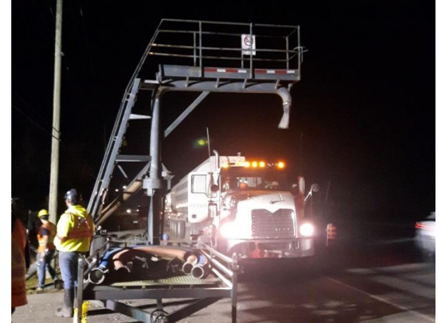
AEGD English church pumping station
