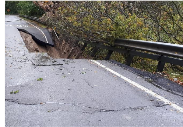
Hwy 8 Dundas Escarpment Failure
