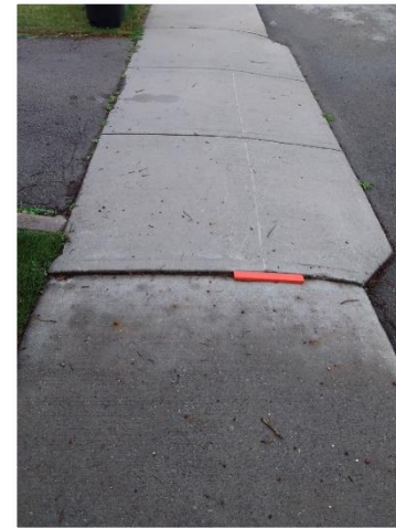
Trip Hazard Deflection
