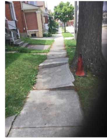
Root Damage Deflection
