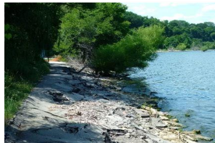
Waterfront Trail damage
