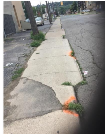
Uneven Surface Deflection 75
