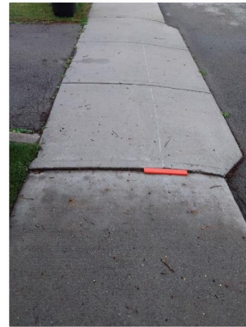
Trip Hazard Deflection
