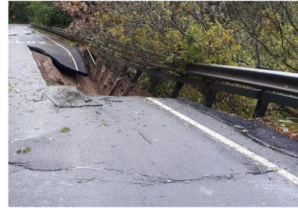
Hwy 8 Dundas Escarpment Failure
