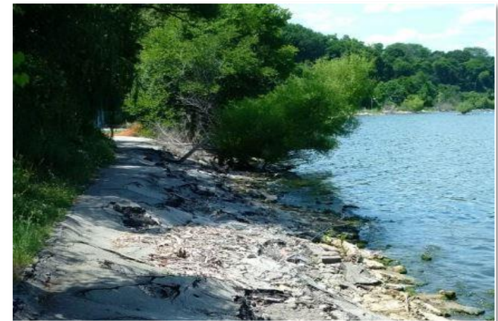
Waterfront Trail damage
