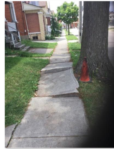
Root Damage Deflection
