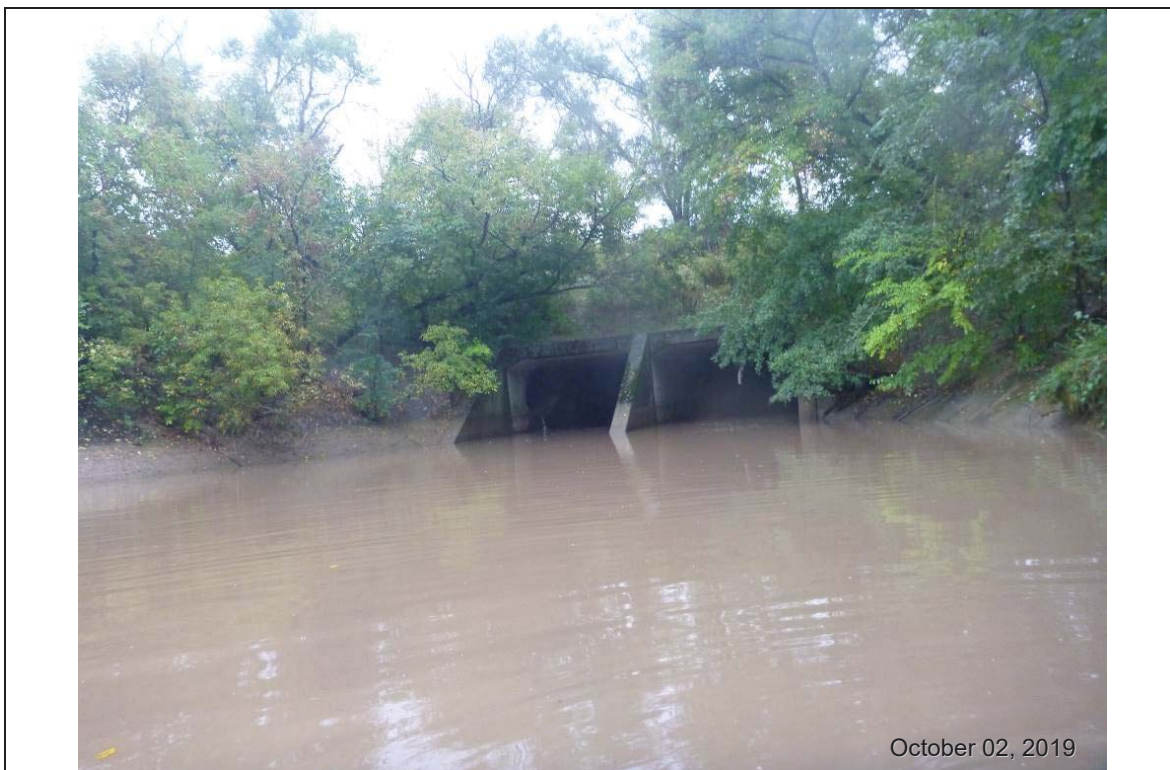
Photograph 3. Steep concrete banks near box culvert at Glen Road and Tope Crescent.
