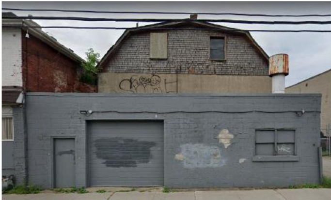
Figure 10: The foreground is a c. 1960s one-storey concrete block entrance at 202 (formerly 200) Cannon Street. In the background is a 19 th century, two storey, gambrel roof abandoned "industrial" building. Source: Google Images.
