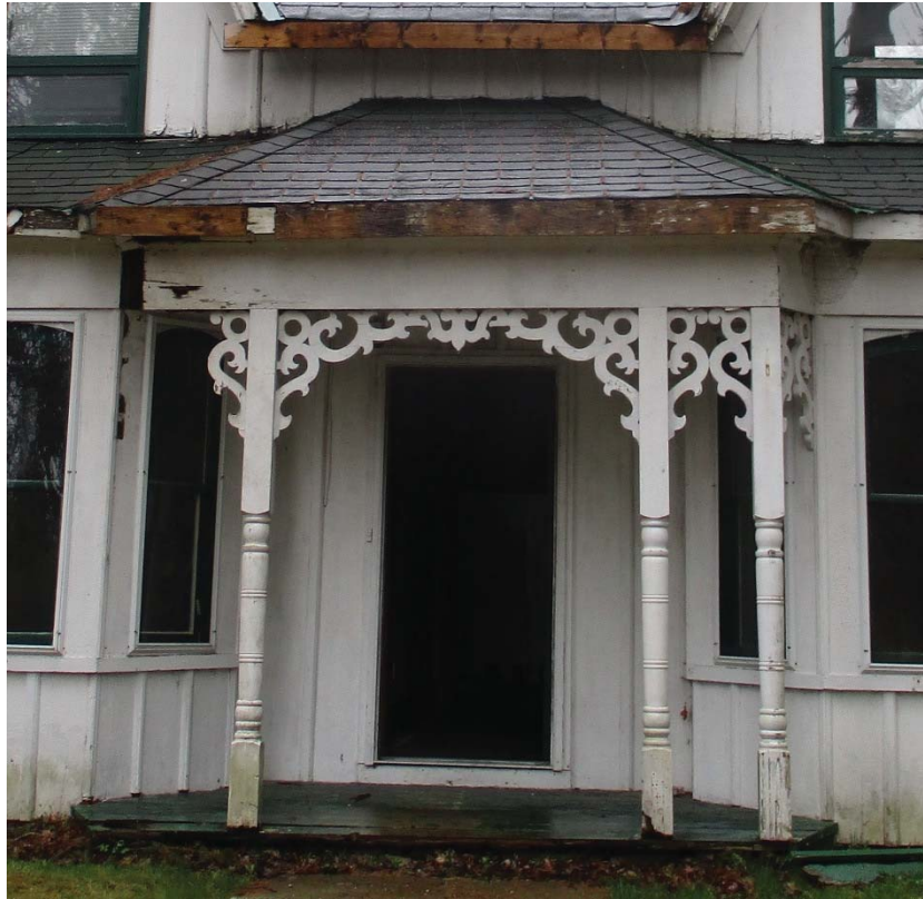
Porch with upside-down posts
