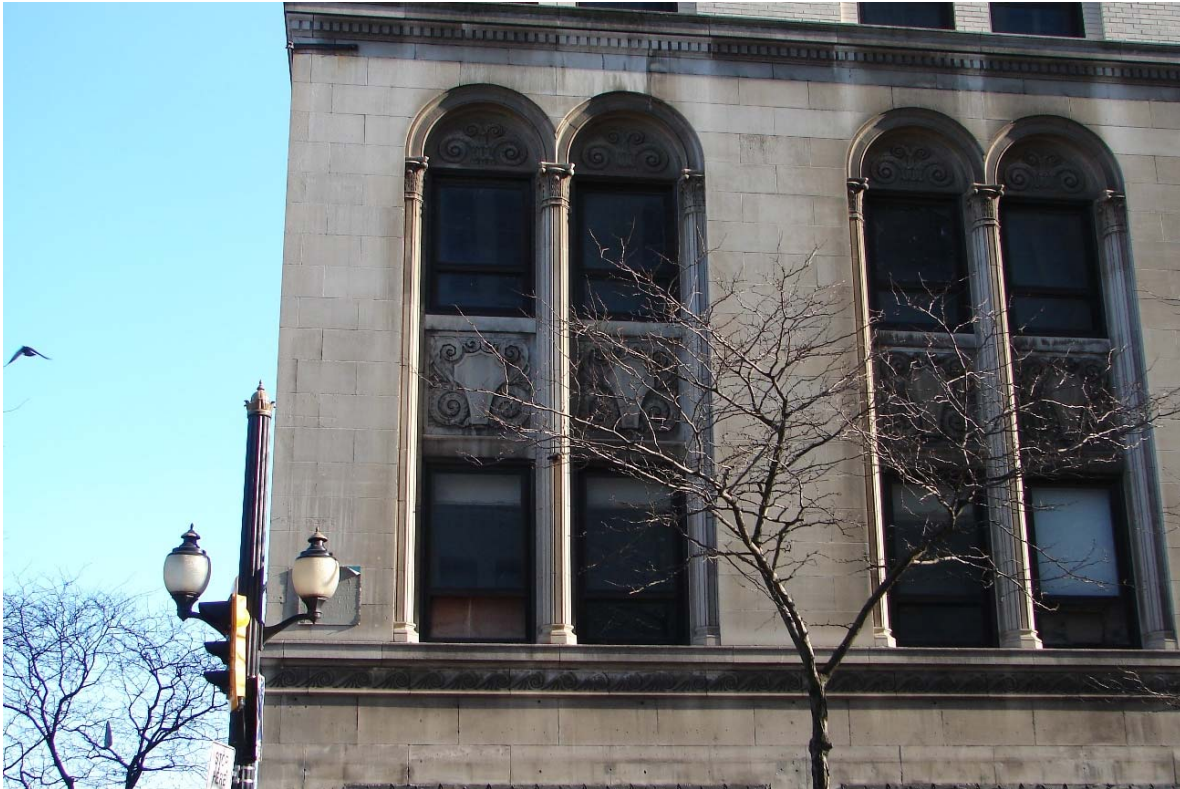
Fig. 74 Window pairs on mezzanine and second floors of west elevation's base (note also dentils in cornice above)
