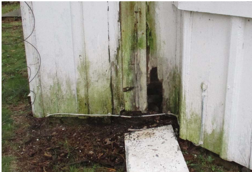
Hole rotted through wall, grade too high
