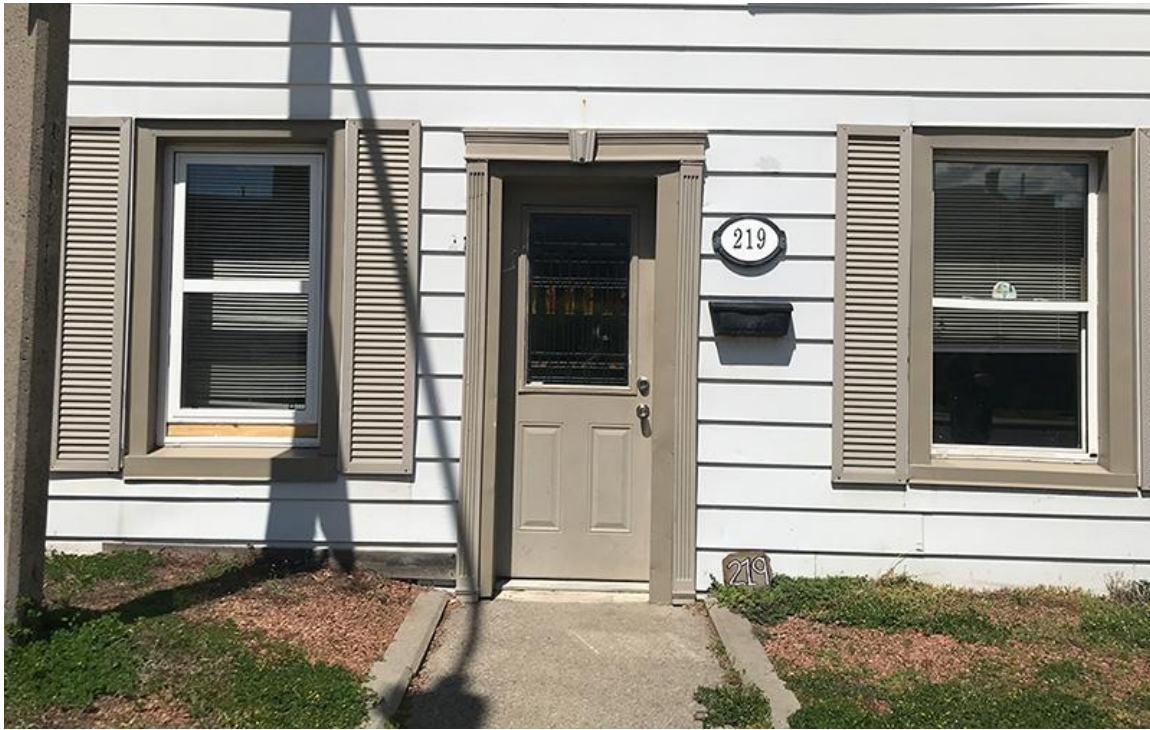
Close-up view of the front doorway and two first storey windows showing the aluminum cladding of the original wood door and window surrounds and a replacement metal door. May 2021
