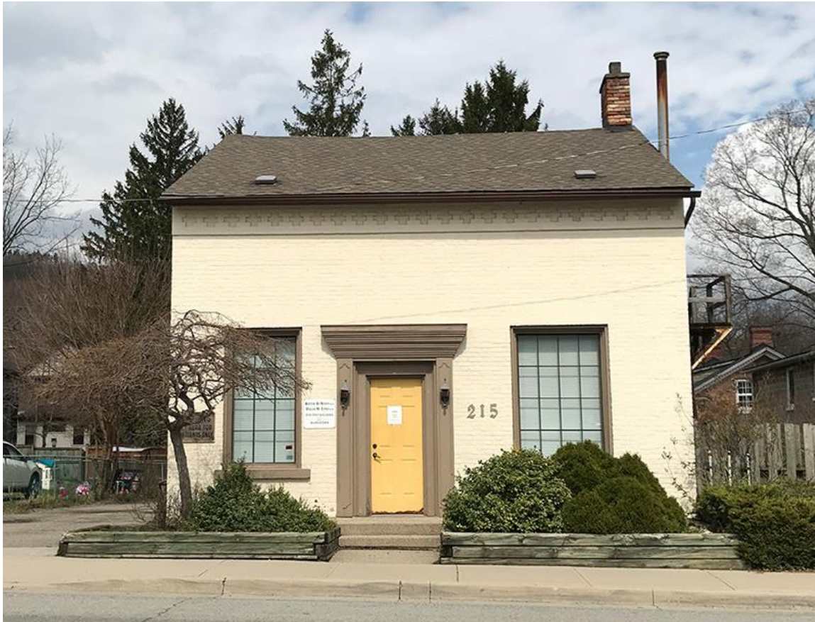
Front (south) façade of #215 showing the decorative course of brickwork below the eaves, and the altered front doorway and windows (thermopane replacements with fake mullions). Photo credit: Ann Gillespie, March 2021
