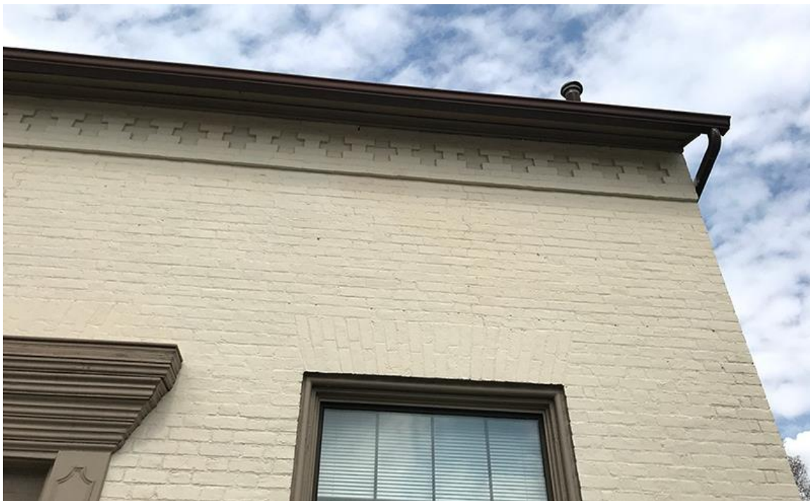
Close-up view of the decorative band of raised brickwork with the cross motif. Also shows the Flemish bond brickwork of the front façade and the flat voussoir arched window and door lintels. The door lintel is largely obscured by the added wood lintel and pilasters. Photo credit: Ann Gillespie, March 2021
