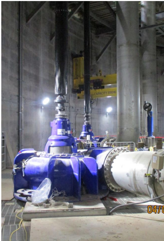
Figure 1: Complete Pumping System Installation
