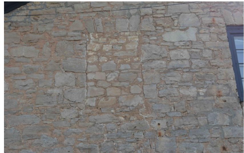
North elevation: eastern-most window opening on 2nd storey has been closed in.
