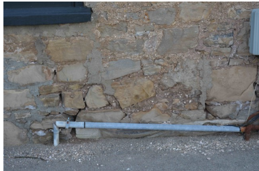
North elevation: failed and open joints, oxidization and metal anchors near foundation.
