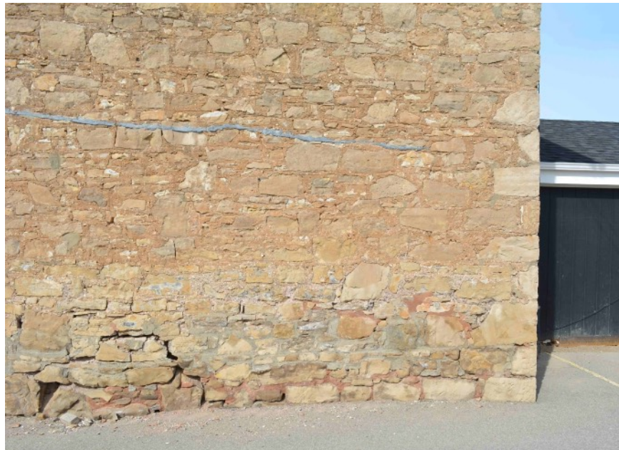
South elevation: failed and open joints at foundation. Movement lines are present at the midsection of this elevation.
