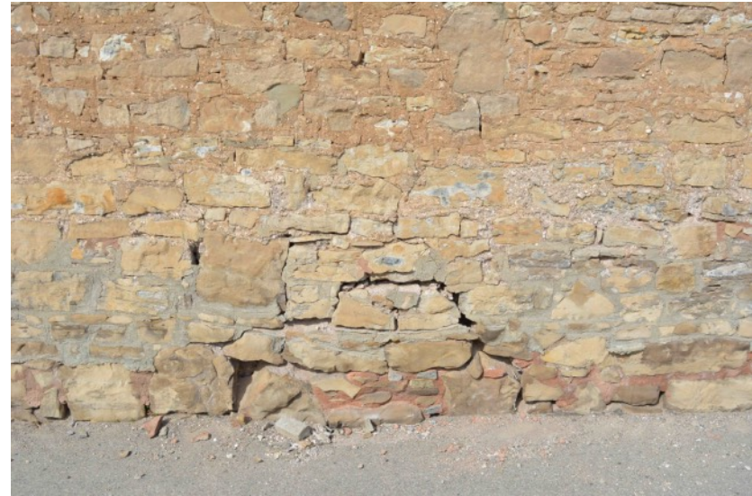
South elevation: ground level failed and open joints with previous repair work also visible.
