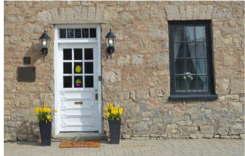
West elevation: Central door with with 12-over-12 sash and five-pane toplight is in good repair.
