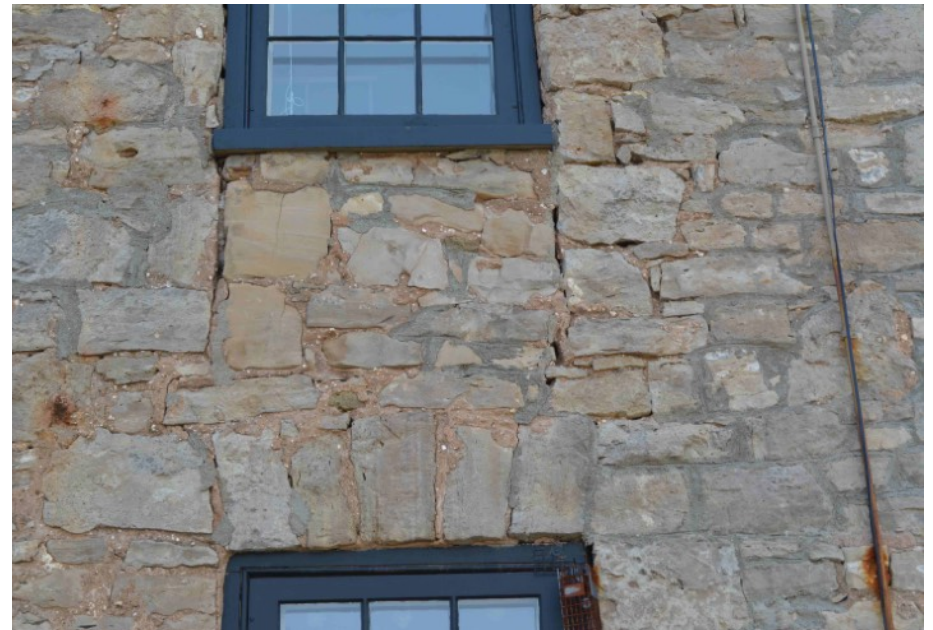
West elevation: Recent repair and pointing work, parging and entire sections of stone removed below the 2nd storey window.
