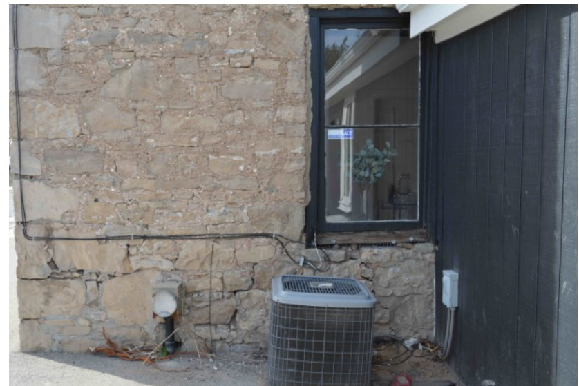
East elevation: Openings at rear elevation have been obscured by the later addition of a one-storey tail.
