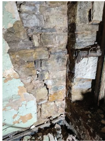
Fig 2: 18-20, 2 nd floor, West return wall separation
