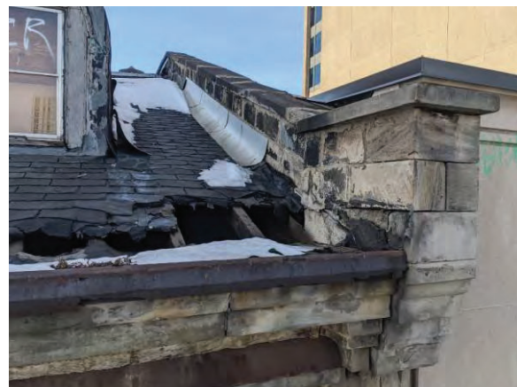
Fig 4: 18-20. Failed roof, pier at upper corner of façade
