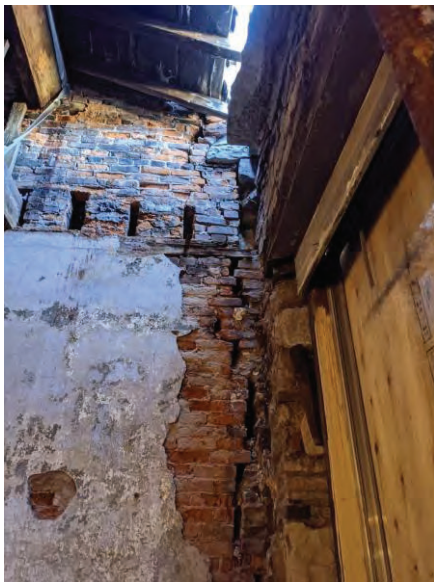
Fig 1: 18-20, 3 rd floor, West return wall separation
