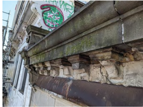
Fig 13: Deteriorated stone below cornice.
