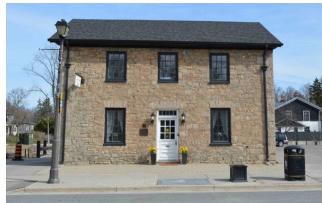
Marr House, 2021 (GBCA). West Elevation 2.4 meters from Wilson Street East. Although the designation by-law notes that chimneys are a contributing heritage attribute, in its current state these are no longer present.
