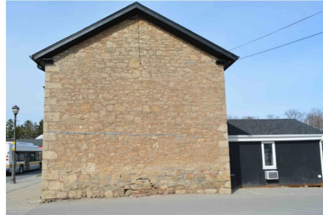
Marr House, 2021 (GBCA). South Elevation. Blank wall with tail extending to the east. Foundation issues notable from a distance.
