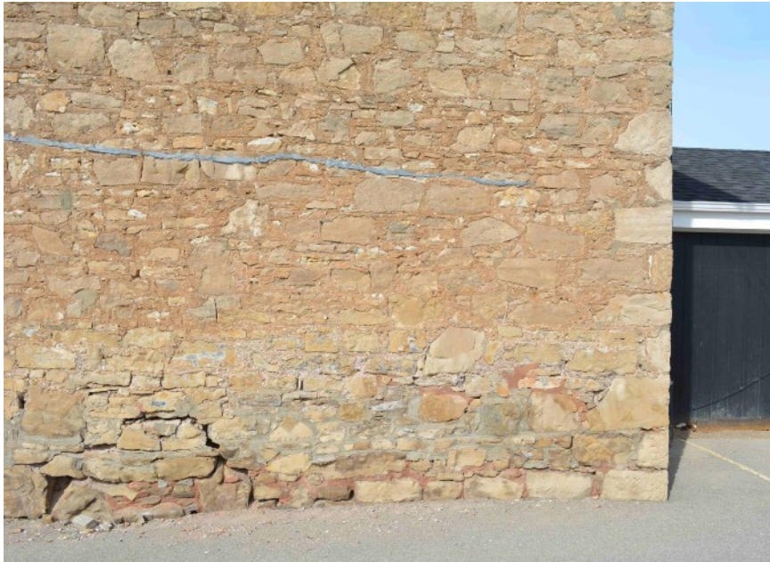
South elevation: failed and open joints at foundation. Movement lines are present at the midsection of this elevation.
