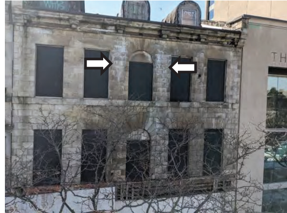
Fig 6: 18-20, upper façade, efflorescence noted
