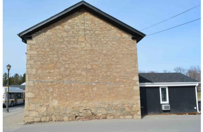
Marr House, 2021 (GBCA). South Elevation. Blank wall with tail extending to the east. Foundation issues notable from a distance.
