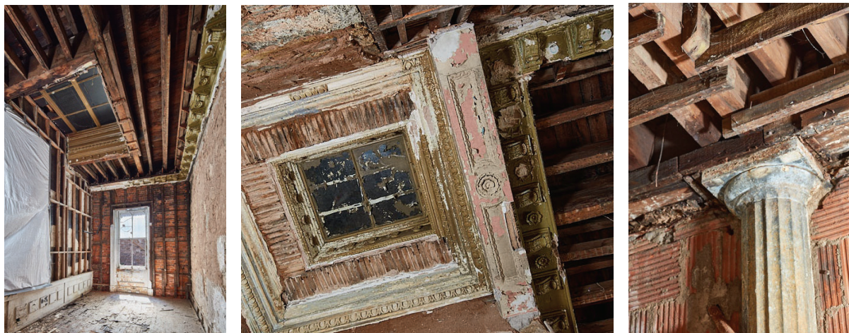
18-22 KING E (THE KERR BUILDINGS) – photo-documentation of ornamental plasterwork and Doric columns on the 1 st floor revealed during remediation work
