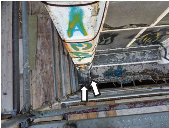
Fig 17: 28 King, E-most pier, looking down, note rotation, and gaps
