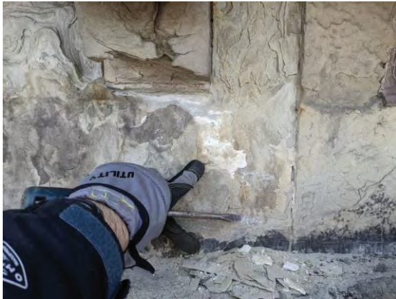
Fig 14: Subflorescence and stone flaking
