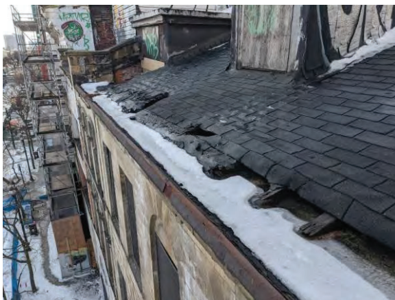
Fig 3: 18-20, failed roof rotted framing above cornice
