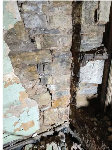
Fig 2: 18-20, 2 nd floor, West return wall separation
