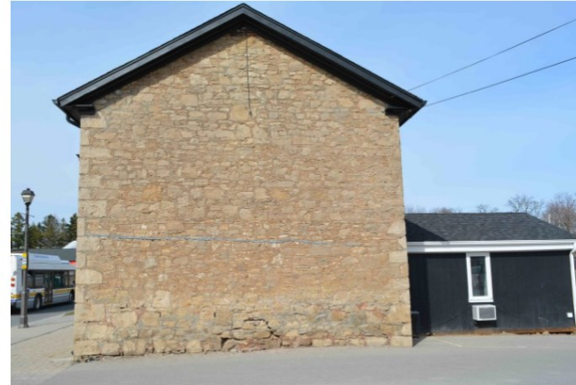
Marr House, 2021 (GBCA). South Elevation. Blank wall with tail extending to the east. Foundation issues notable from a distance.
