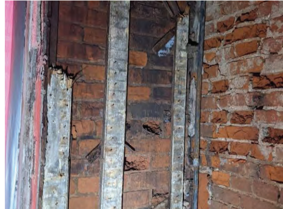
Fig 16: 24 King, saturated, deteriorated brick.
