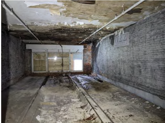
Fig 15: 24 King, 3 rd floor level, severe water damage.
