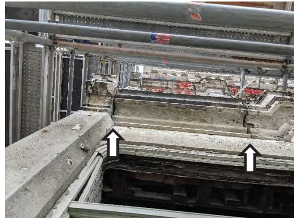
Fig 18: 28 King, E-most pier/spandrel, looking up note gaps in head joints.
