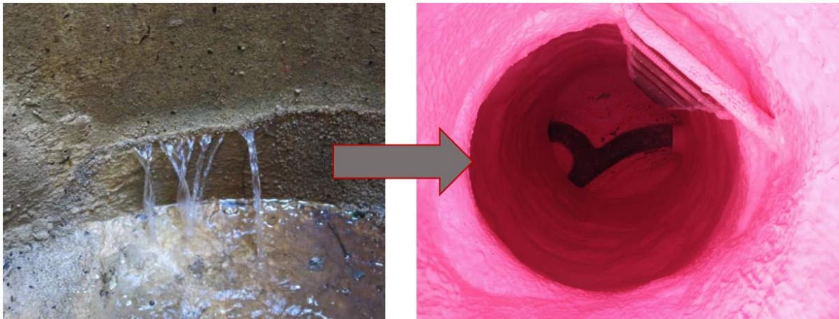
Figure 1.2: Infiltration in Manhole (left) and SpectraShield® Sealant in Manhole to Mitigate Infiltration (Right)
