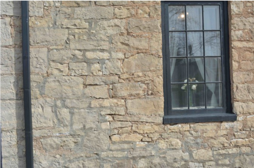
West elevation: ground level showing cementitious parging applied at the northern edge of the building.
