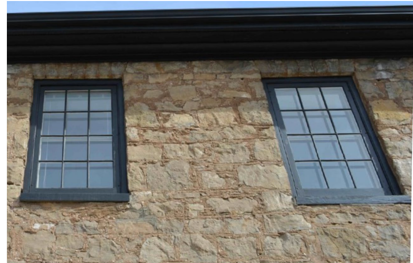
West elevation: window frames on 2nd storey appear to be in good repair upon visual review..
