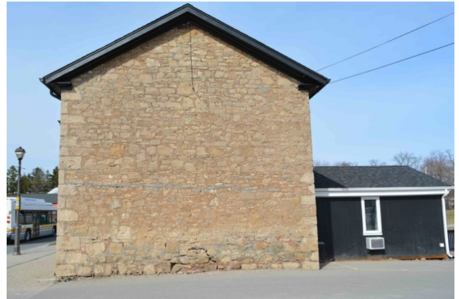
Marr House, 2021 (GBCA). South Elevation. Blank wall with tail extending to the east. Foundation issues notable from a distance.
