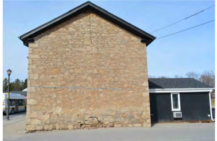
Marr House, 2021 (GBCA). South Elevation. Blank wall with tail extending to the east. Foundation issues notable from a distance.
