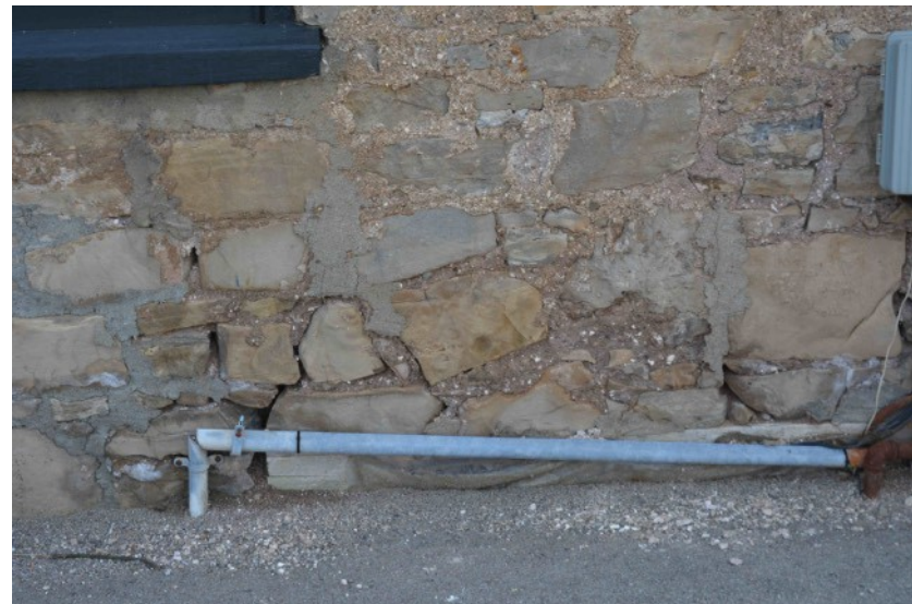
North elevation: failed and open joints, oxidization and metal anchors near foundation.
