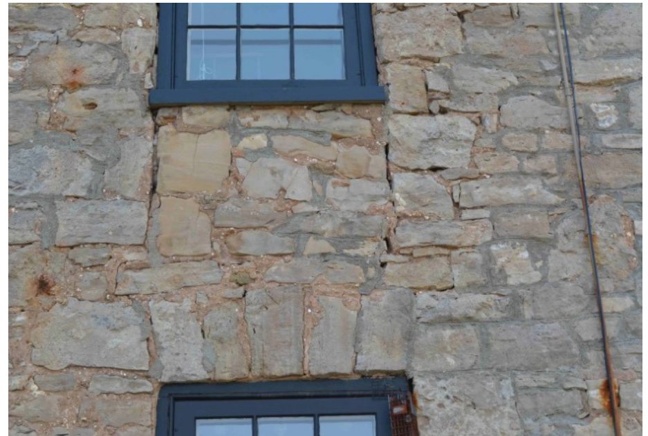
West elevation: Recent repair and pointing work, parging and entire sections of stone removed below the 2nd storey window.
