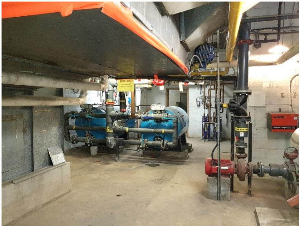
Figure 70: Mechanical/filtration room, looking west. All equipment has been replaced over time.
