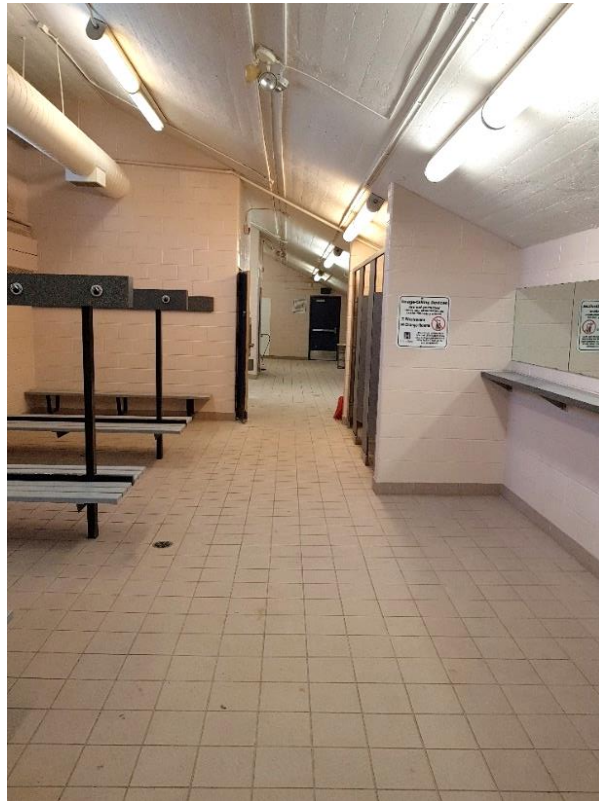
Figure 52: Female change room, looking north. Note slope in ceiling from pool bleachers.
