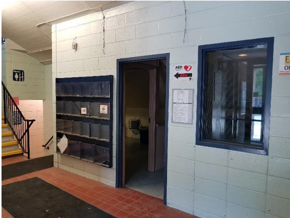
Figure 37: Looking northwest at entrance to office rooms and stairs leading up to the pool floor and stairs leading down to the ground floor.
