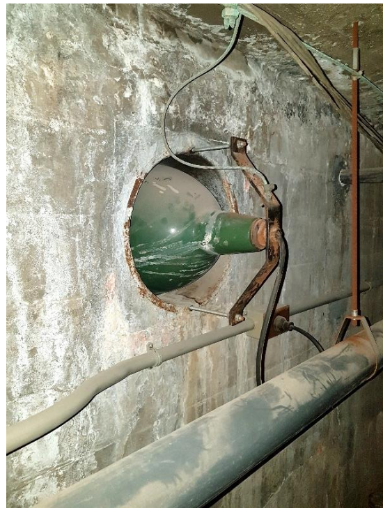
Figure 72: Under water pool light; this light appears to be original. Note, marks of the board forms are visible on the cement.
