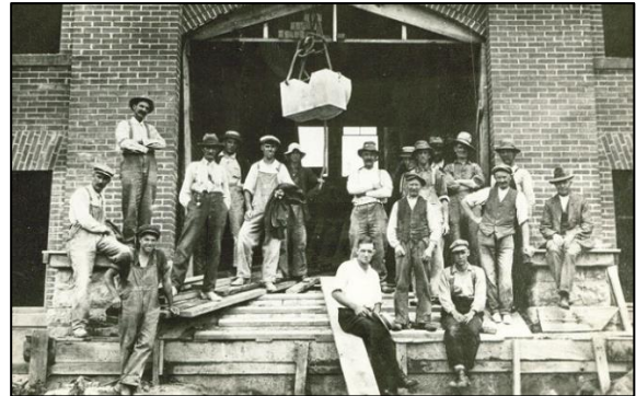
Figure 38: Waterdown Public School under construction in 1921 (Flamborough Archives, BW 186, C. A. Newell Collection)
