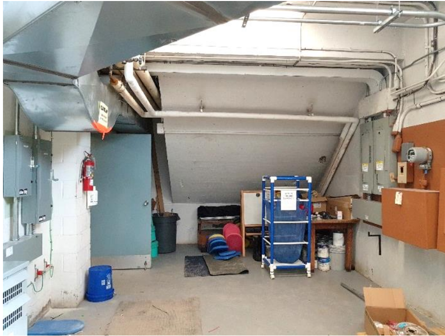
Figure 51: Electrical room, looking north.
