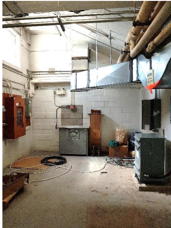
Figure 50: Electrical room, looking south. Enclosed in 1974/75 to create a designated electrical room.
