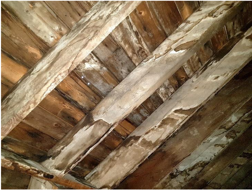
Figure 87: Roof deck on the frontispiece appears to be constructed in tongue and groove method.
