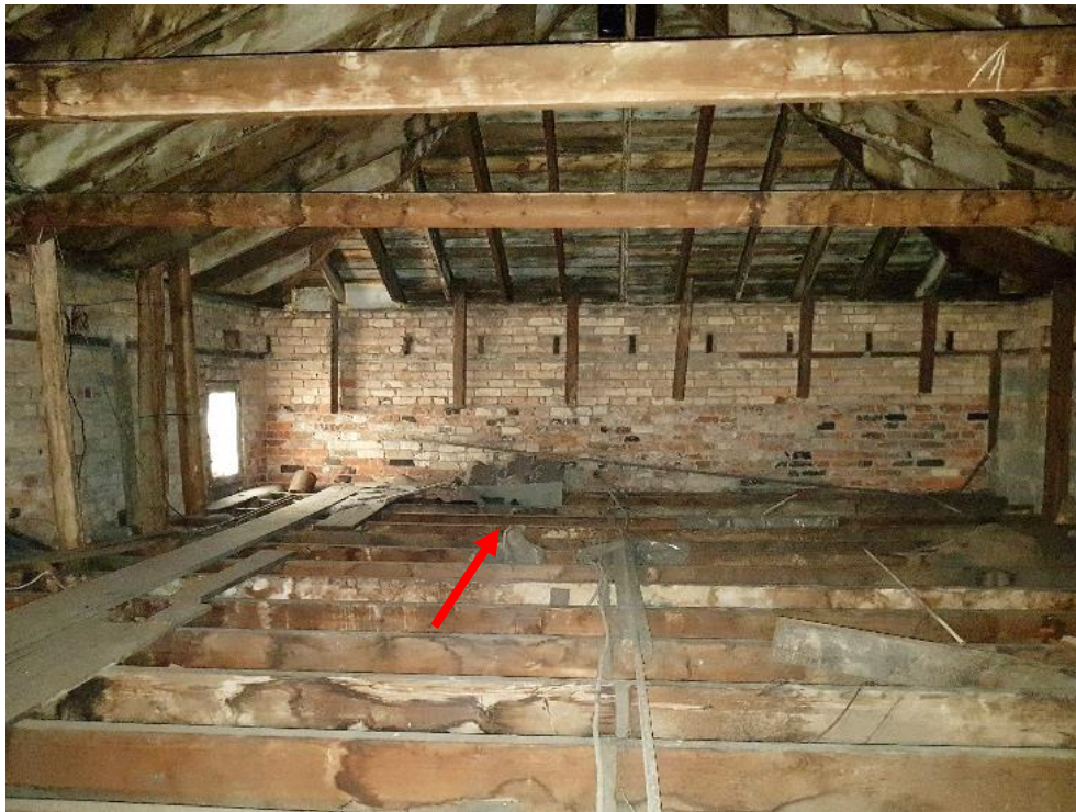
Figure 83: Looking east within the attic space of the frontispiece. The arrow points to red roof tiles, which may be the original to the frontispiece.
