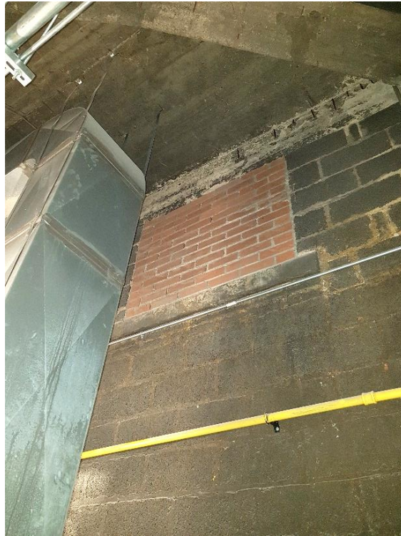
Figure 67: Ground floor: covered window within a/c room along west wall, looking west.
