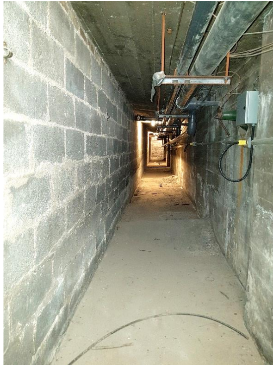
Figure 71: Pipe tunnel that runs around the perimeter of the pool. Note, electrical and pipes within pipe tunnel has been updated.
