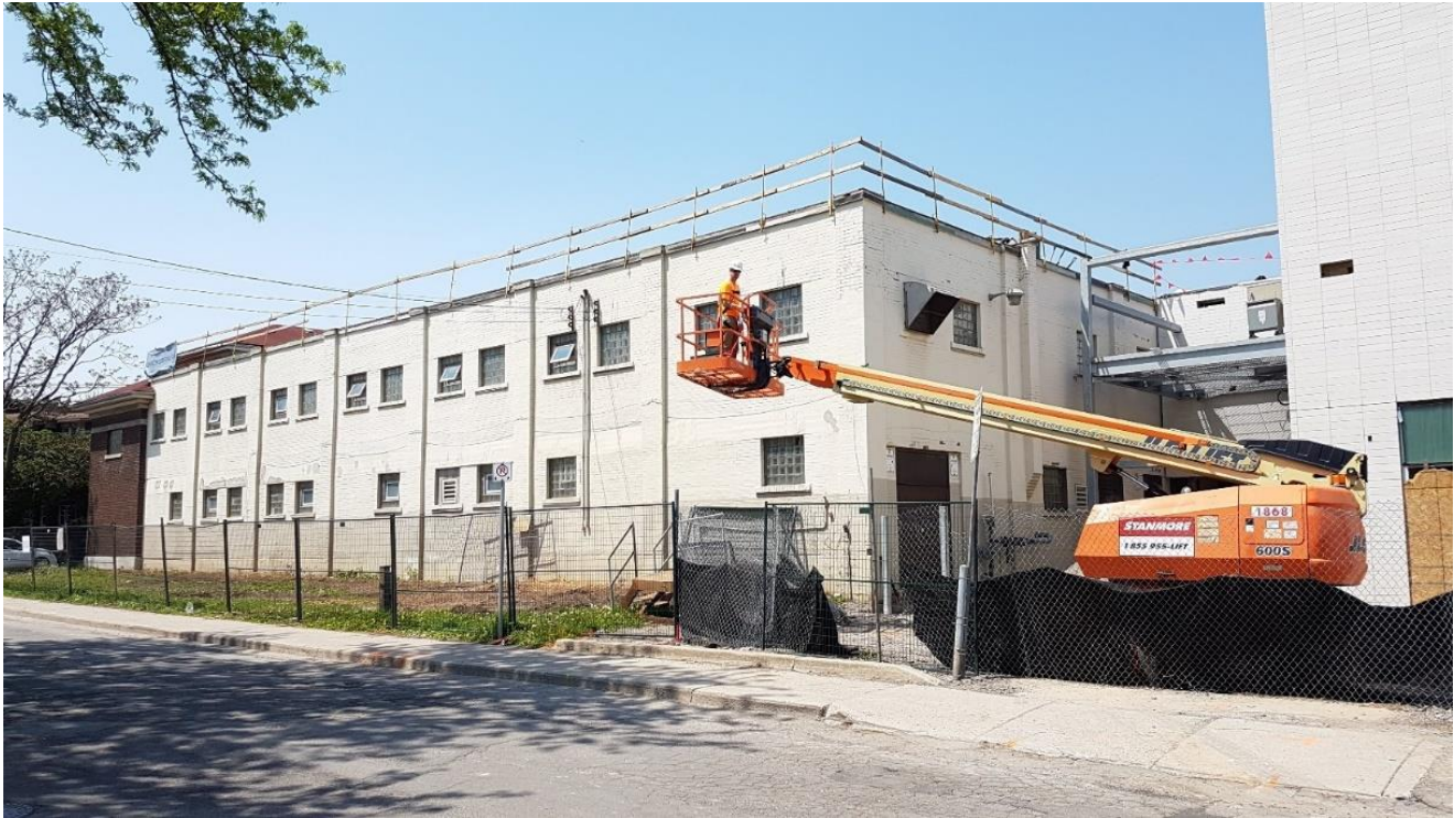
Figure 31: Looking southwest at the east and north facades of the Jimmy Thompson Memorial Pool.
