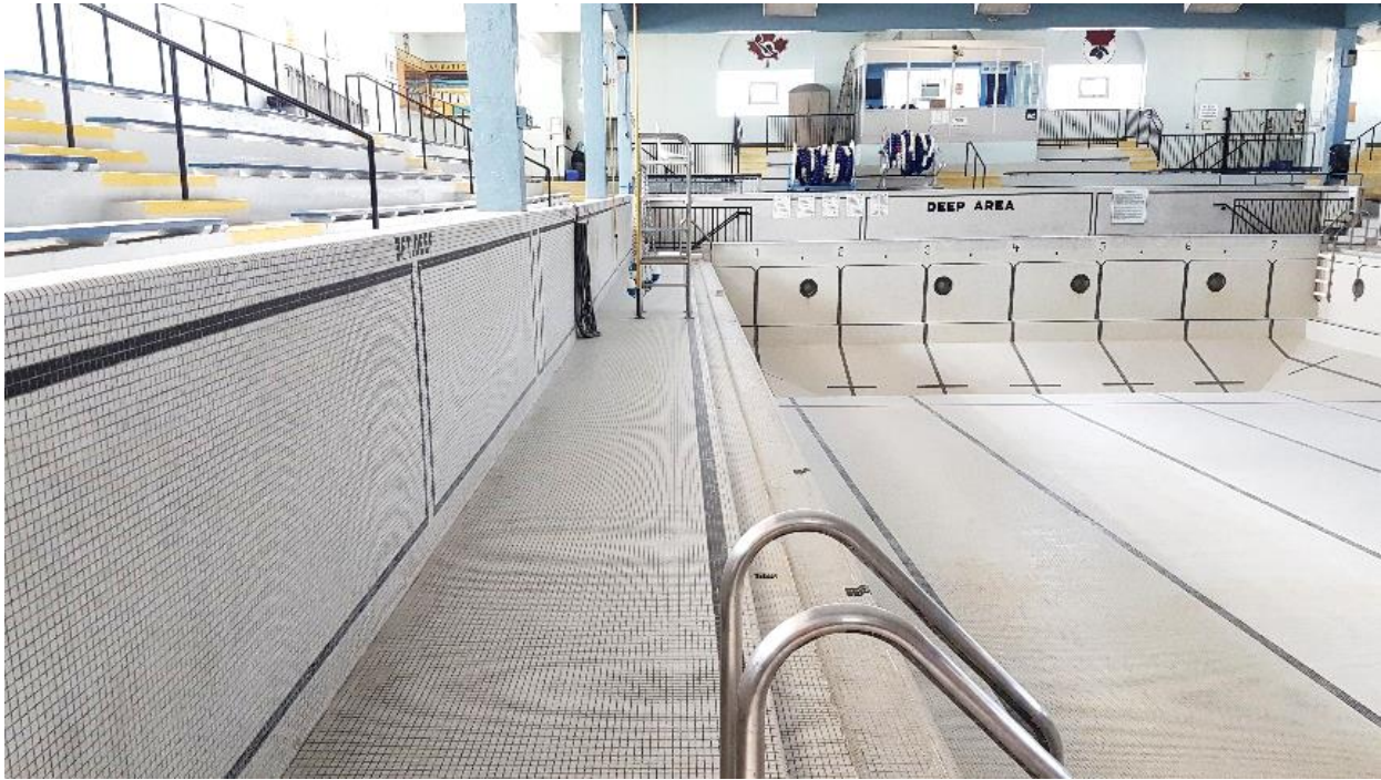
Figure 77: Wall separating bleachers from the deck level, looking south. Gutters are visible between the deck and pool.
