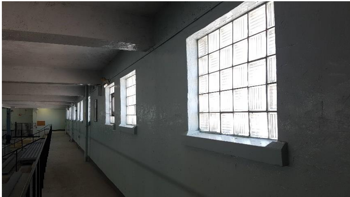
Figure 76: Updated glass-block windows along west side of pool. Note, some of the windows are fitted with a centre single-hung opening.
