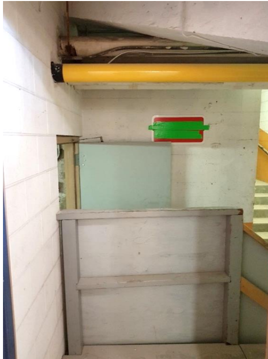
Figure 61: Stairs from corridor to a/c room, emergency exit and mechanical/filtration room. Note, stairs from corridor to subsequent rooms were constructed in 1974/75 when the wall was opened, looking north.
