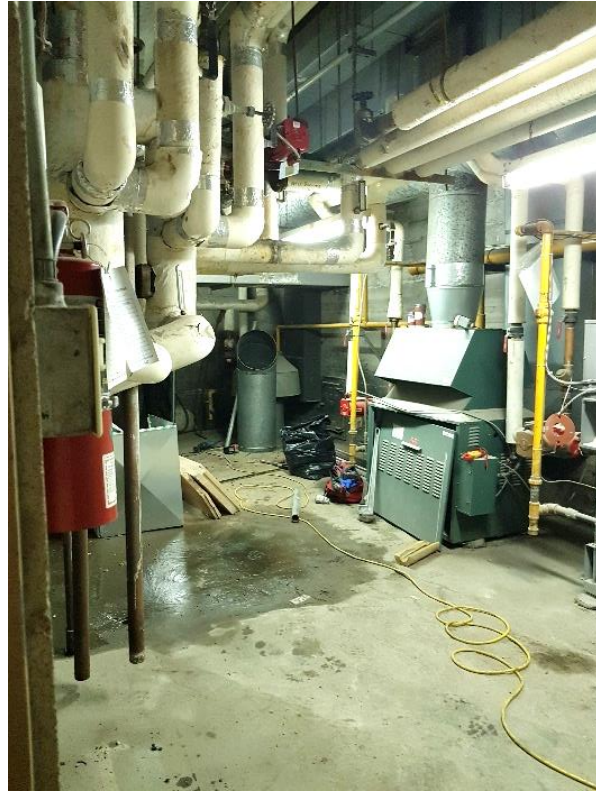
Figure 63: Furnace room, looking south west. All equipment has been updated over time.
