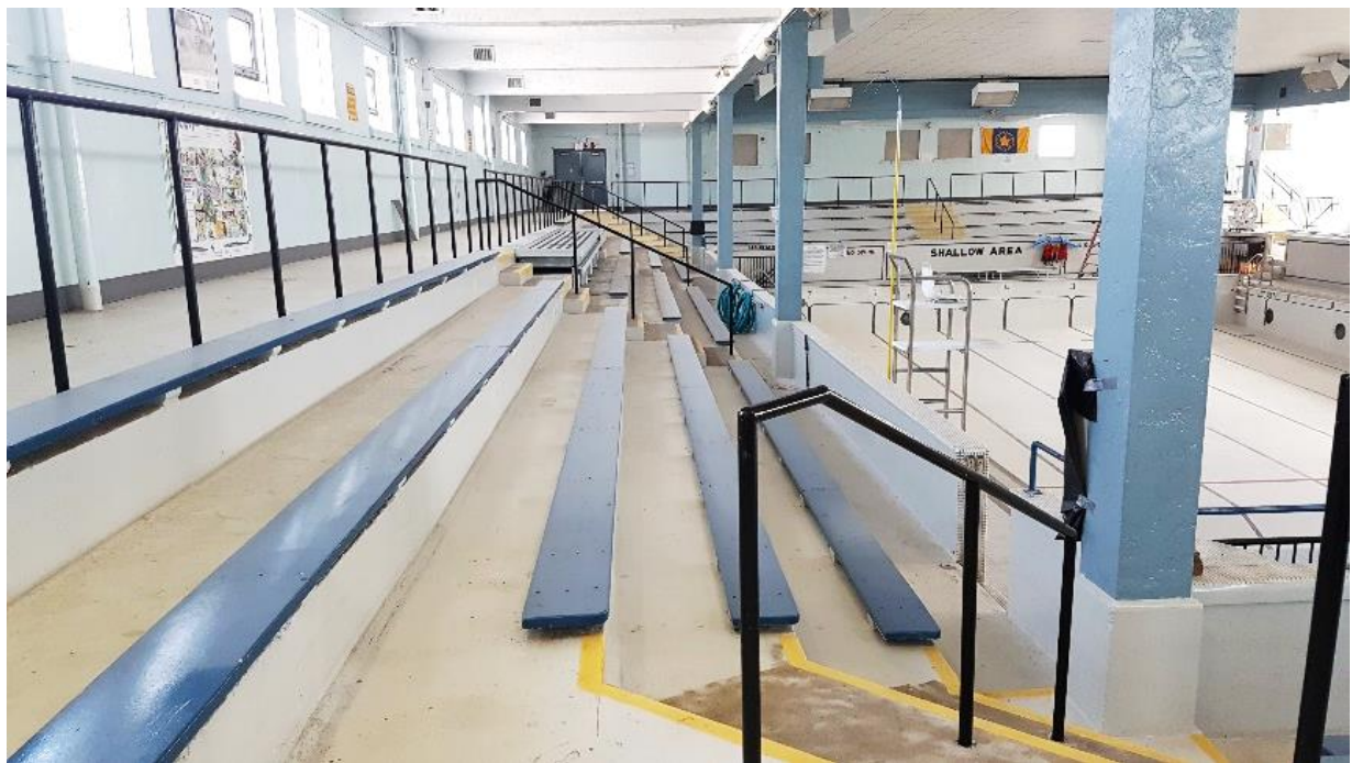
Figure 74: Bleacher rows along the west side of the pool, looking north. Note, the absence of the Corinthian capitals and decorative base on the columns. Roof columns are evident. The drop ceiling over the former skylight is visible.
