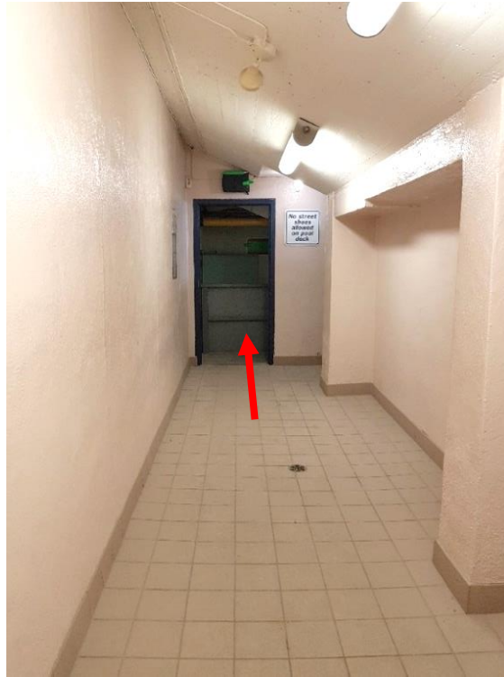
Figure 59: Corridor north of female change room, looking north. Wall at north end was opened and a door installed in 1974/75 for access to an emergency exit.
