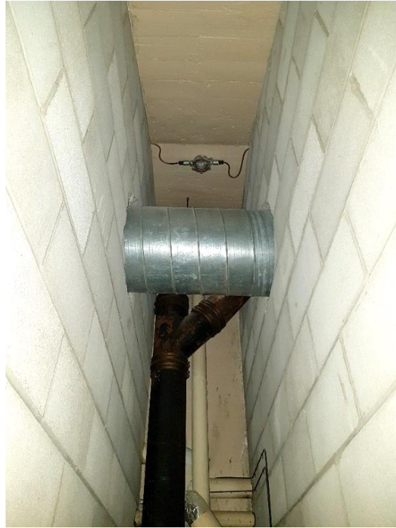
Figure 55: Air vent within utility room of the female change room, looking west and up.
