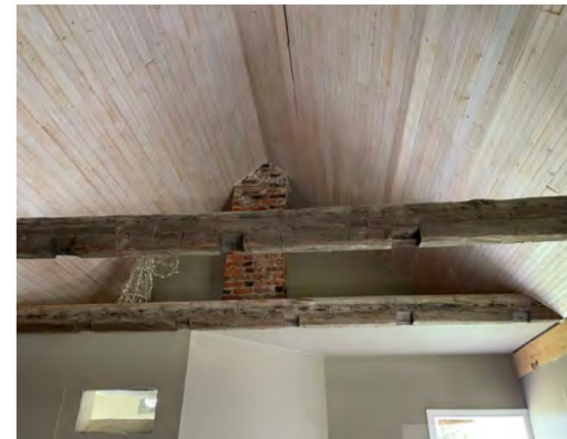
Fig. 5.19. Example of new ceiling and beams; Beams are not original to this house and were salvaged from another property
