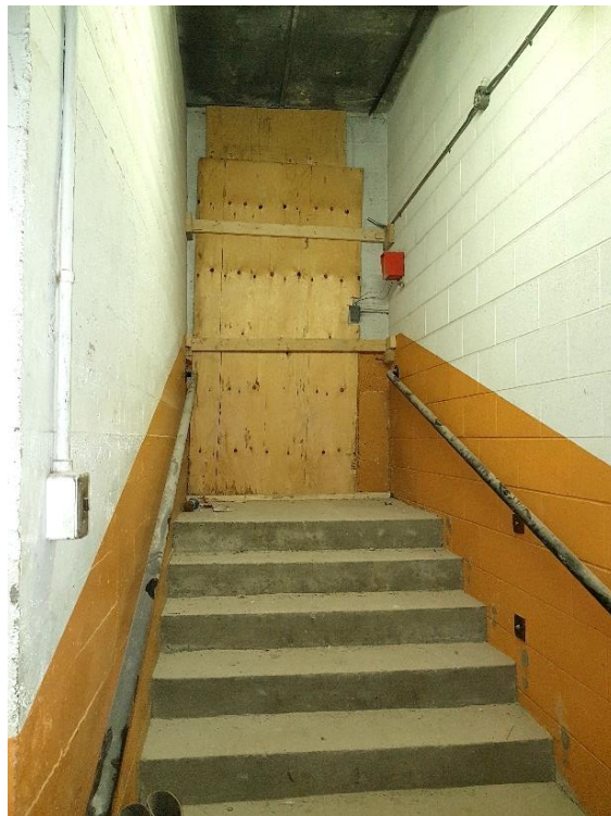
Figure 68: Rear exit, which was utilized as an emergency exit from the female change room after 1974/75, looking north.
