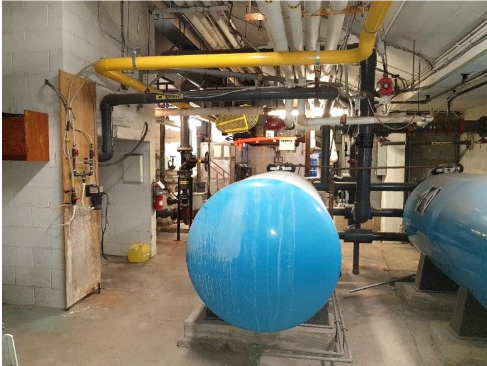
Figure 69: Mechanical/filtration room, looking east. All equipment has been replaced over time.
