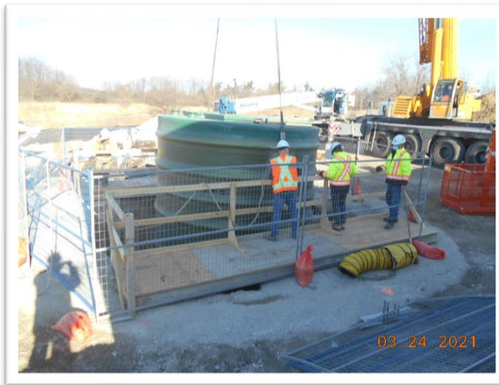
Twenty Road Wastewater Pumping Station
