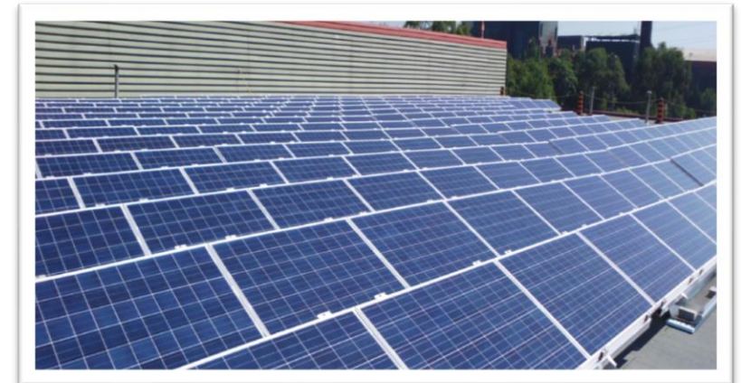
Solar Panels at 330 Wentworth
