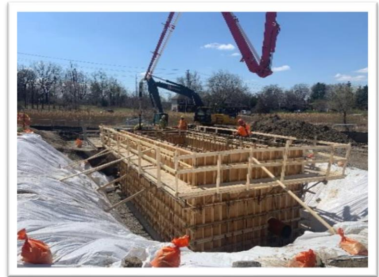
Twenty Road Wastewater Pumping Station
