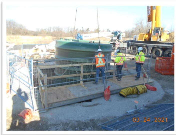
Twenty Road Wastewater Pumping Station
