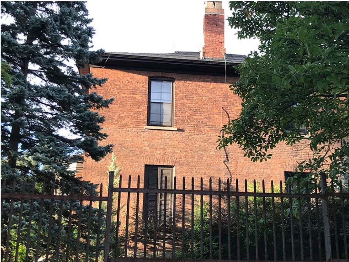
South façade of 2-storey addition showing the voussoir-arched brick window lintels and stone sills.
