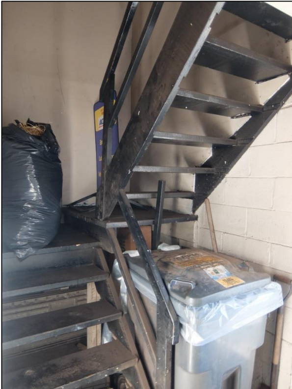
Image 14: Metal stairwell to upper-floor (private residence) above the commercial office, December 2021 (City of Hamilton)
