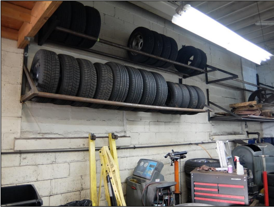
Image 13: Second interior garage bay in rear addition looking north to former exterior concrete-block rear wall of the original building (now an interior wall) and blocked-in window opening with lintel, December 2021 (City of Hamilton)
