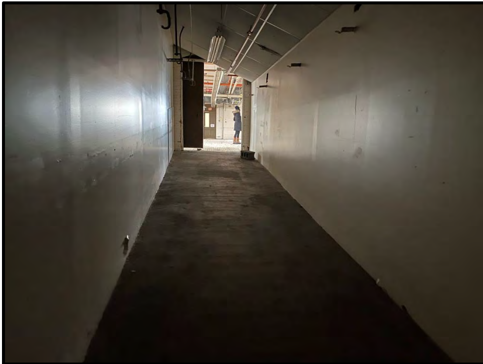
Image 142: Fourth Floor Ramp to Brick Building – Interior (Photo taken on December 8, 2021; Facing West)
