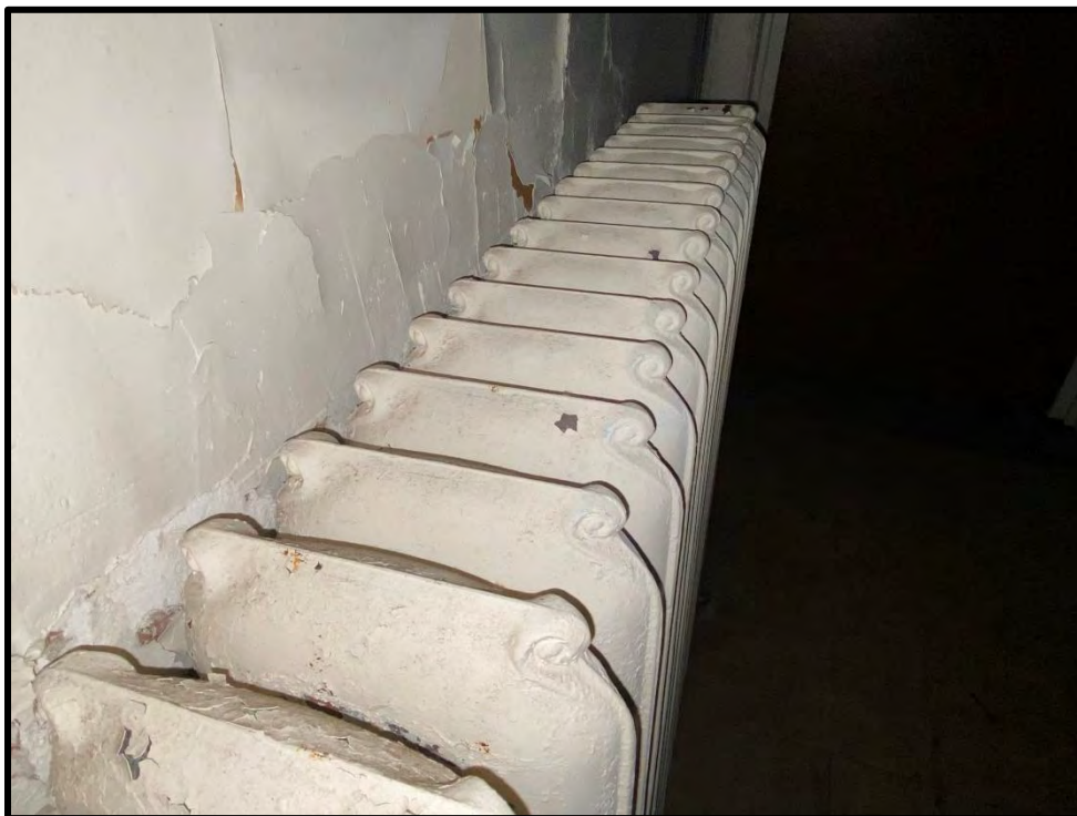
Image 94: First Floor North Addition – Stairwell Radiator (Photo taken on December 8, 2021)
