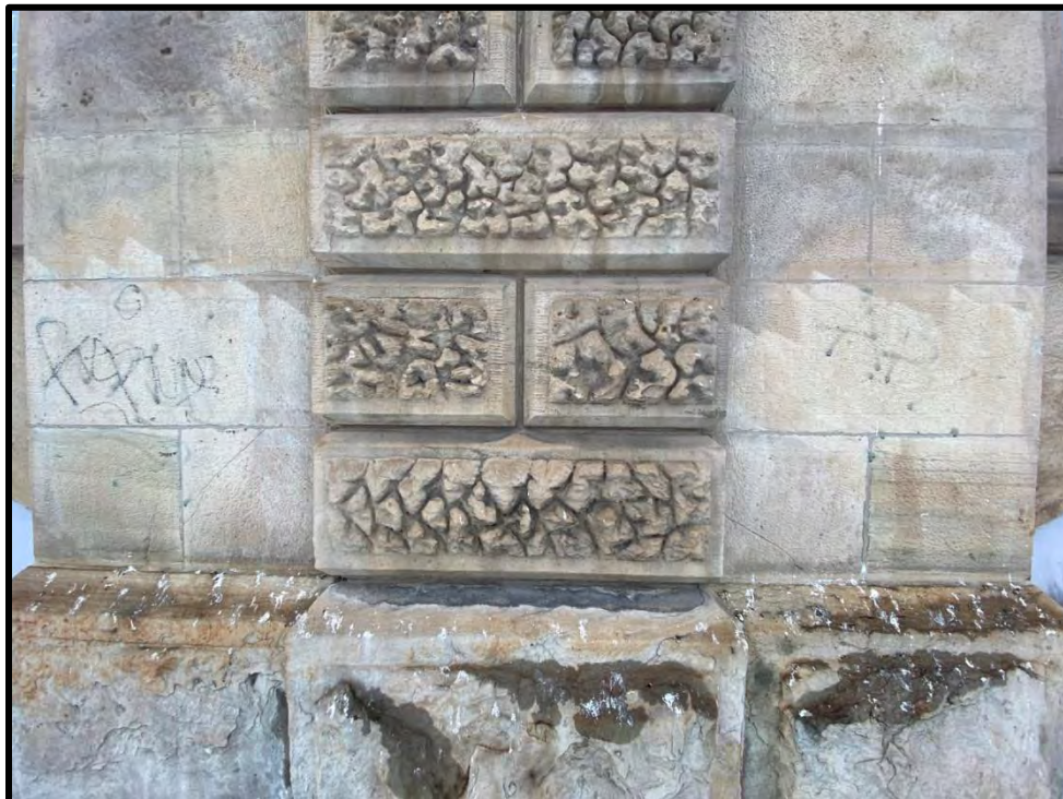
Image 10: Vermiculated Stone Pilaster and Dressed Stone – Detail (Photo taken on December 8, 2021; Facing North)
