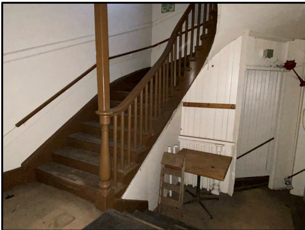
Image 96: First Floor North Addition – Stairwell and Basement Entrance (Photo taken on December 8, 2021)
