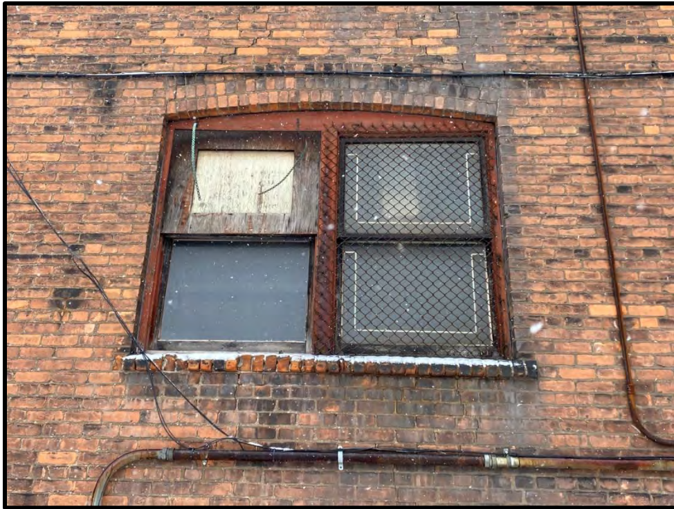
Image 51: Window Opening on North Elevation – Detail (Photo taken on December 8, 2021; Facing South)
