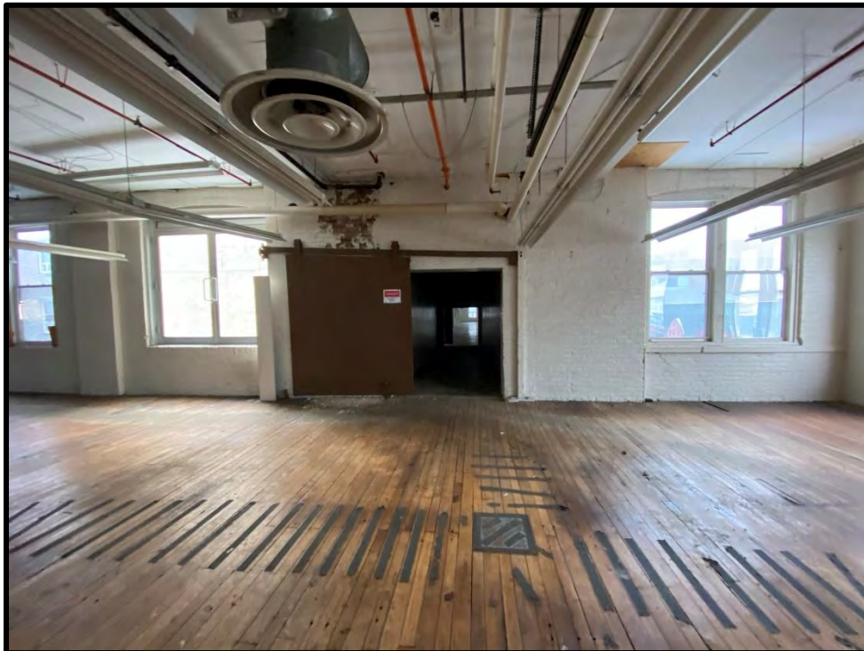
Image 170: Second Floor Brick Building – Opening to Stone Building (Photo taken on December 8, 2021; Facing East)
