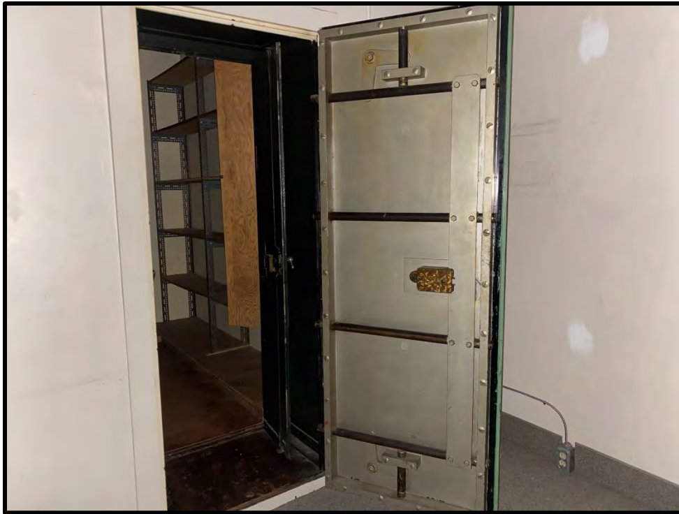
Image 81: First Floor North Addition – Vault Detail (Photo taken on December 8, 2021; Facing Northwest)
