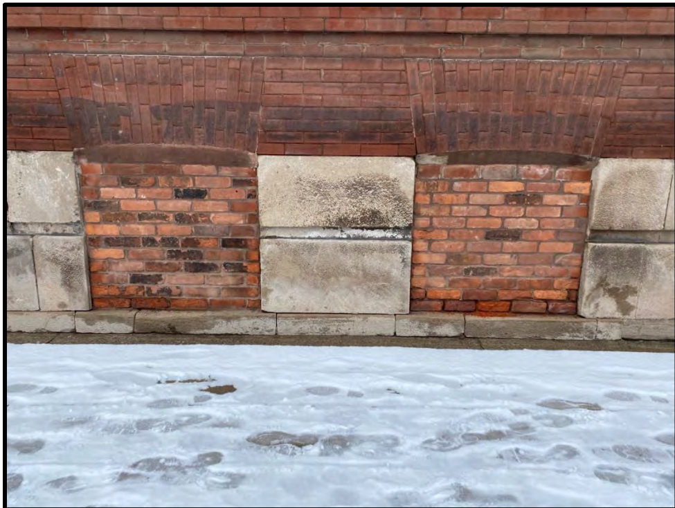
Image 40: York Street Front Façade Basement Window Opening – Detail (Photo taken on December 8, 2021; Facing North)
