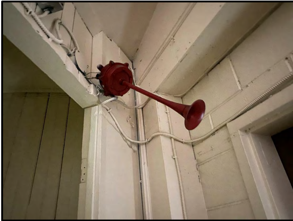
Image 97: North Addition – Basement Entrance Alarm (Photo taken on December 8, 2021)
