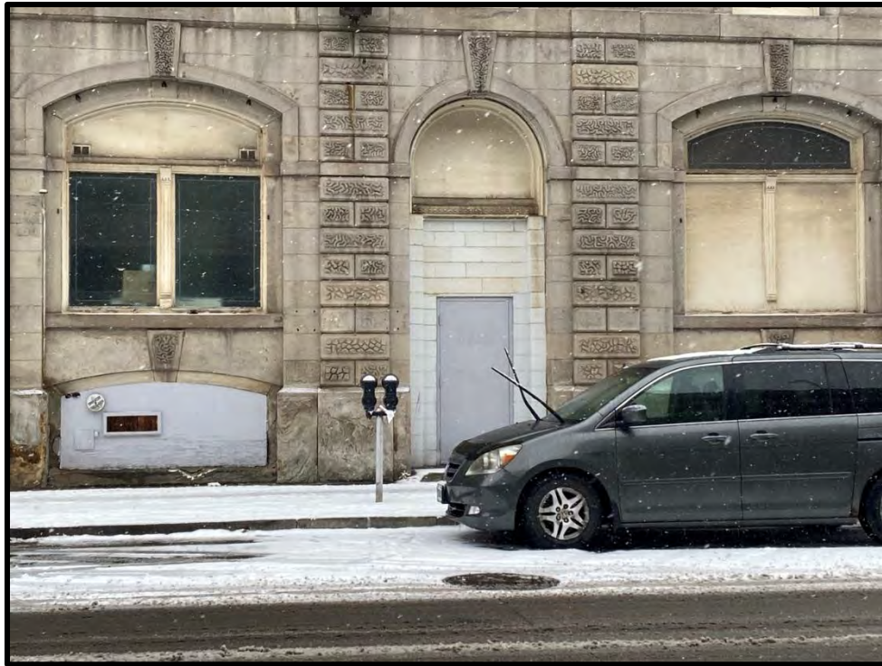
Image 27: East Elevation Window and Door Openings - Detail (Photo taken on December 8, 2021; Facing West)
