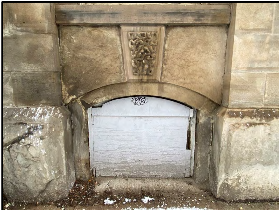
Image 8: Detail of Basement Window Opening on York Street Front Façade (Photo taken on December 8, 2021; Facing North)
