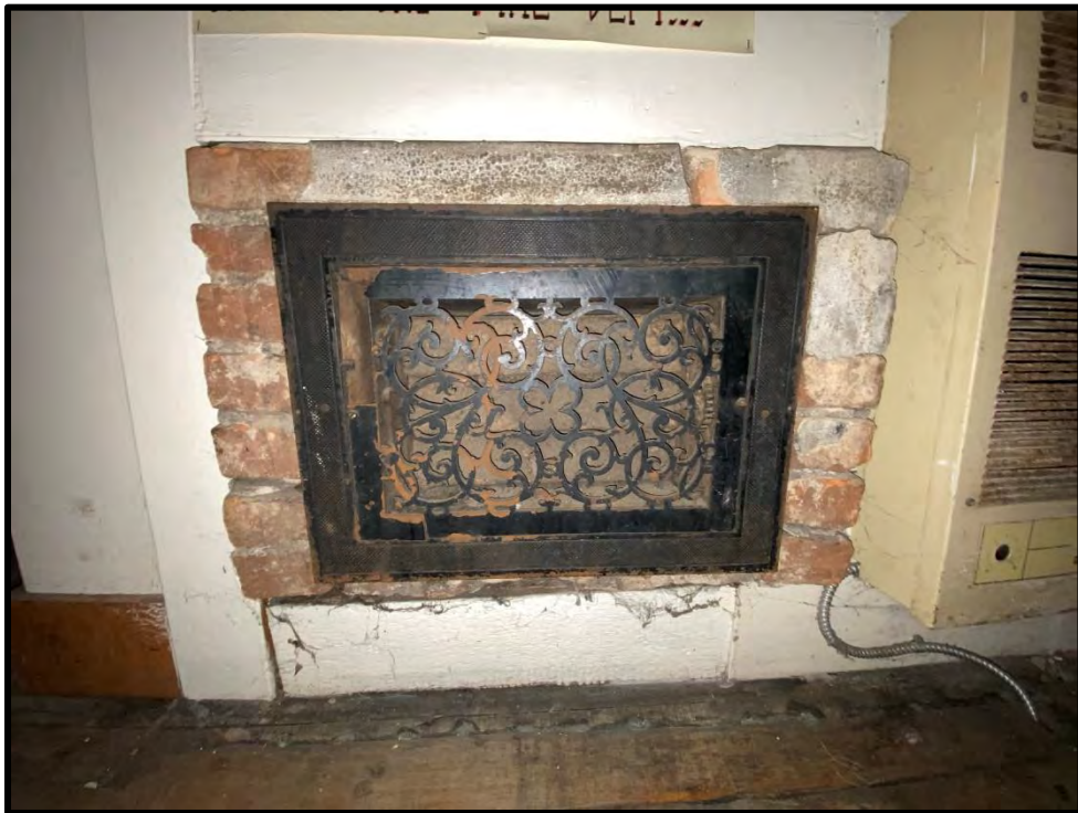
Image 90: First Floor North Addition – Heat Register Detail (Photo taken on December 8, 2021; Facing South)
