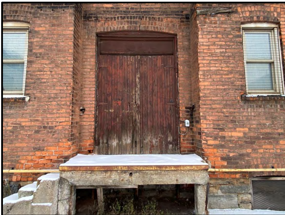
Image 46: Detail of Door Opening on West Elevation (Photo taken on December 8, 2021; Facing East)
