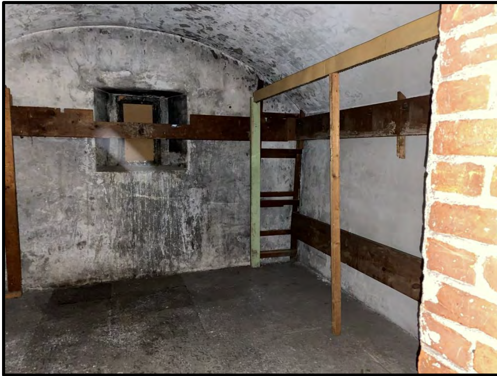
Image 123: Second Floor North Addition Vault – Detail (Photo taken on December 8, 2021; Facing Northwest)
