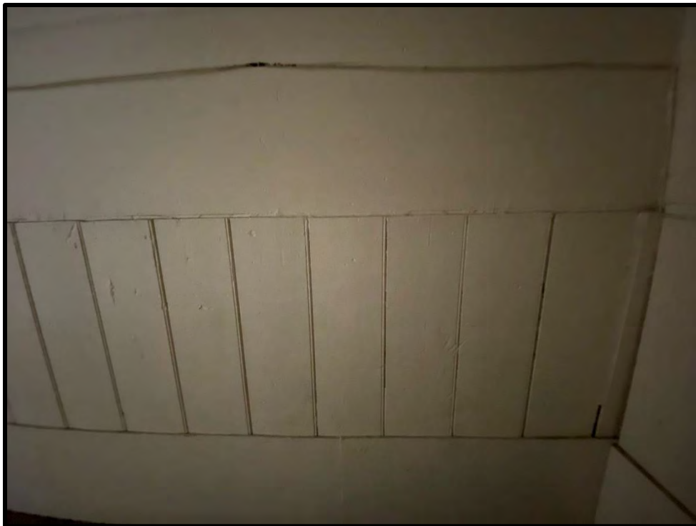
Image 92: First Floor North Addition – Wainscoting Detail (Photo taken on December 8, 2021; Facing South)
