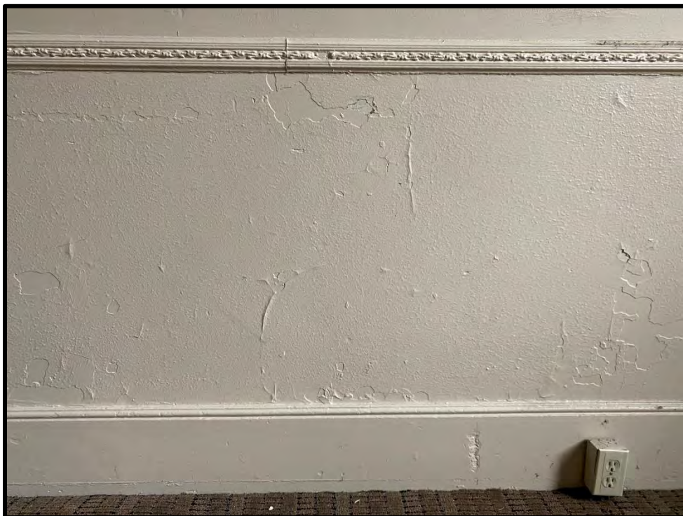
Image 64: First Floor – Interior Detail Chair Rail (Photo taken on December 8, 2021; Facing North)
