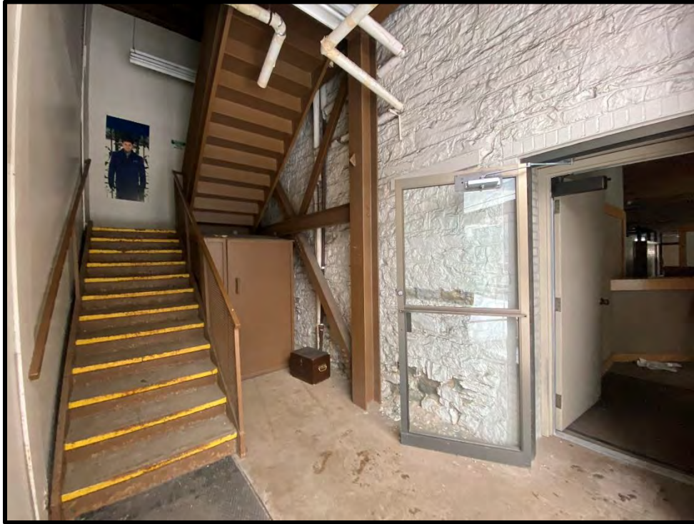
Image 55: First Floor – Stairwell Addition and West Elevation Entrance (Photo taken on December 8, 2021; Facing East)
