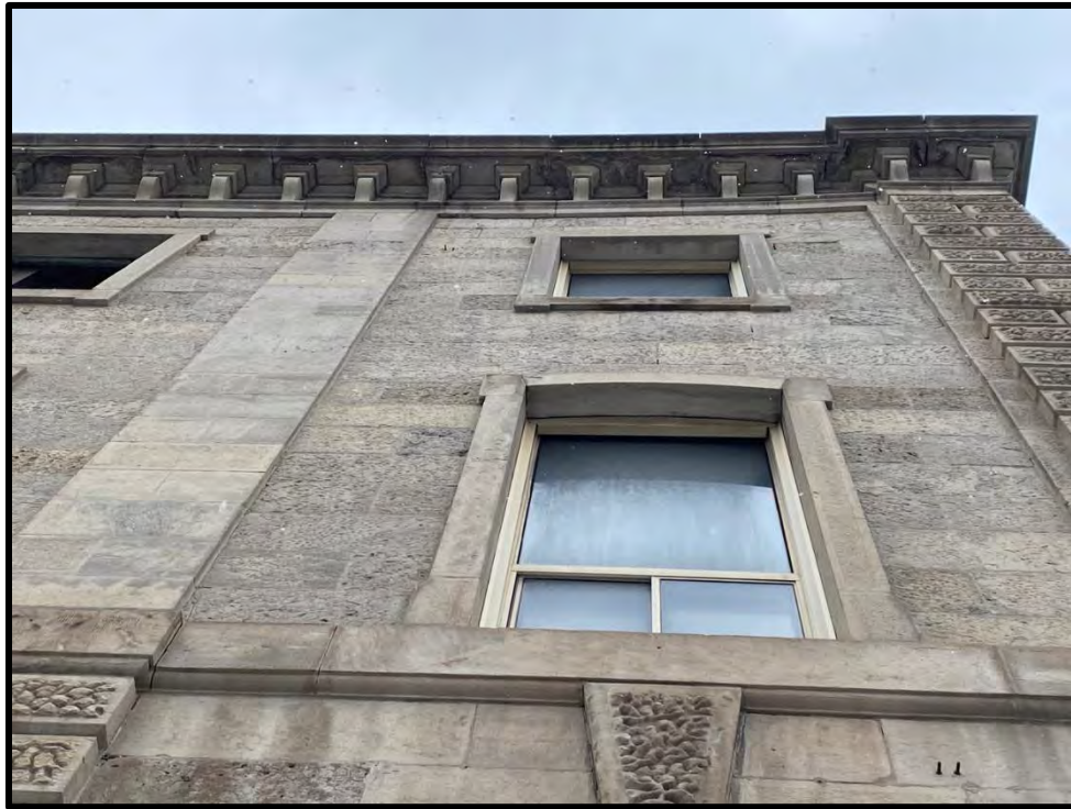
Image 11: Second and Third Storey Window Openings and Brackets – Detail (Photo taken on December 8, 2021; Facing North)
