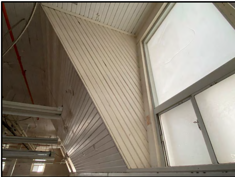
Image 138: Fourth Floor Stone Building – Dormer Detail (Photo taken on December 8, 2021; Facing East)
