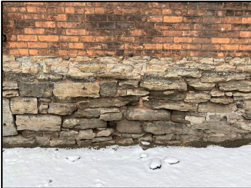
Image 52: Common Bond Brick Coursing and Uncoursed Stone Foundation – Detail (Photo taken on December 8, 2021; Facing South)
