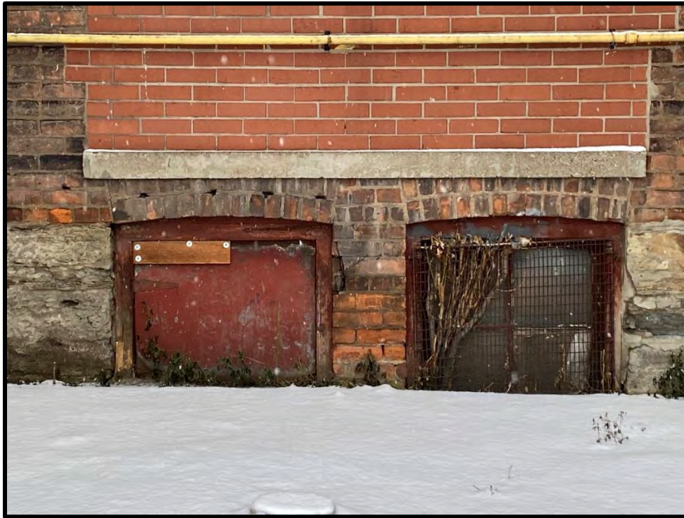
Image 47: Detail of Basement Window Openings on West Elevation (Photo taken on December 8, 2021; Facing East)
