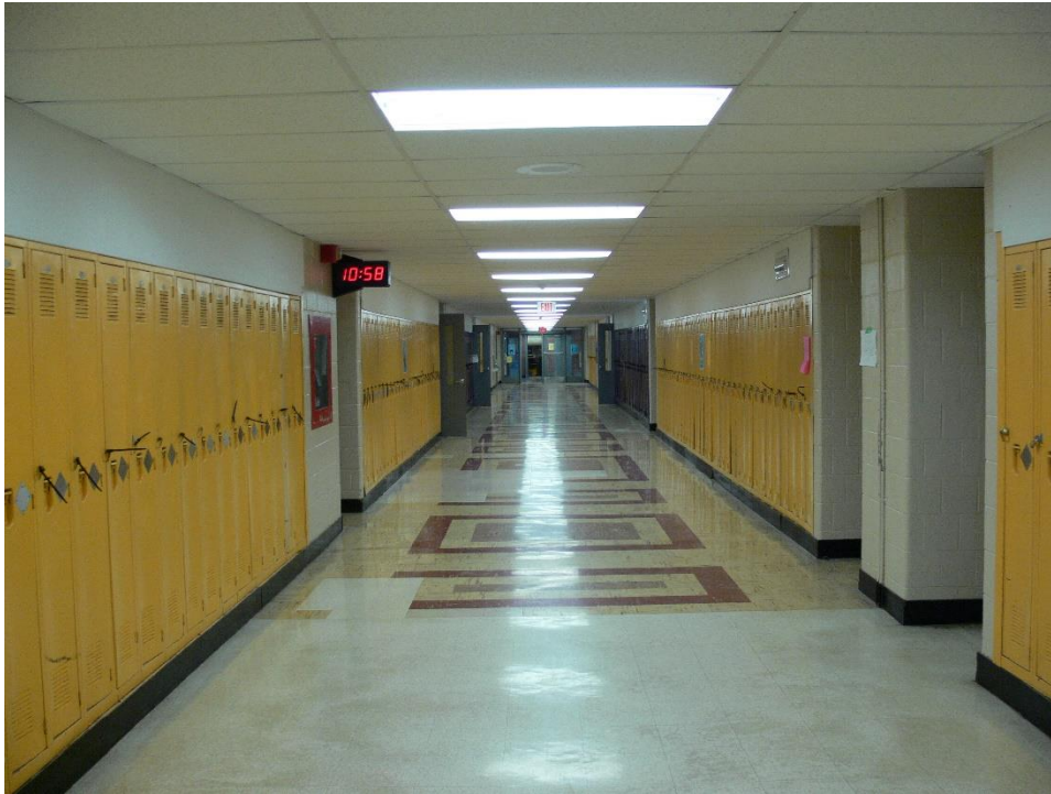
Plate 41: Typical corridor with rust and cream terrazzo featuring patches of linoleum floor replacement
