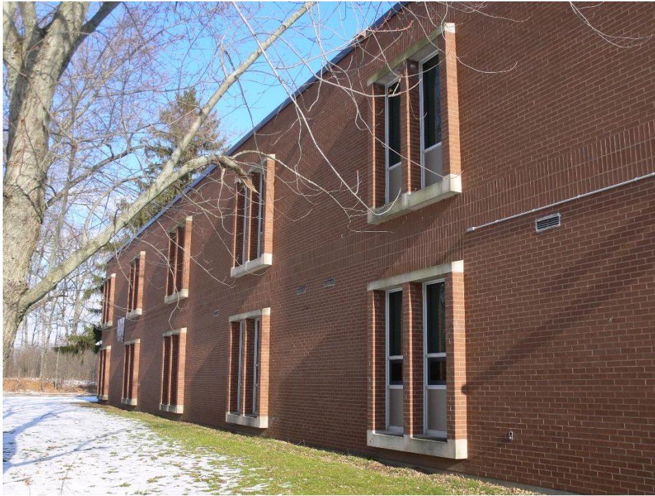
Plate 31: Detail of window surrounds on the west elevation of the West Wing
