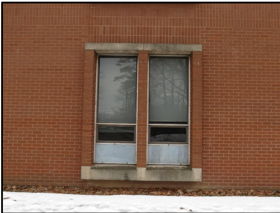
Image 13: Detail of typical paired window, North Elevation of West Wing (Photo taken on March 13, 2019; Facing South)
