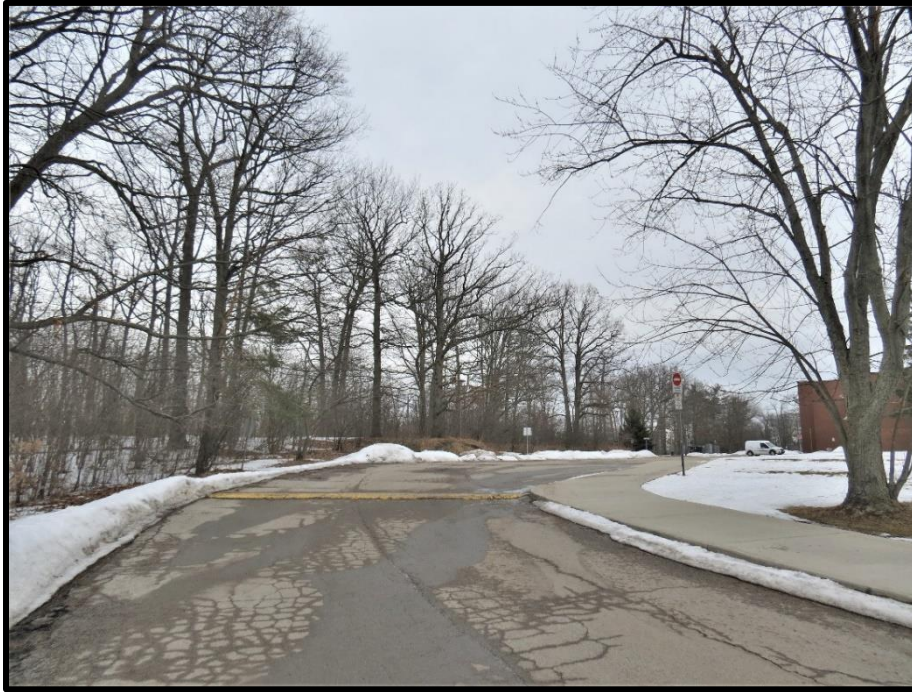
Image 1: View of Private Road across north side – Ancaster High School (Photo taken on March 13, 2019; Facing East)
