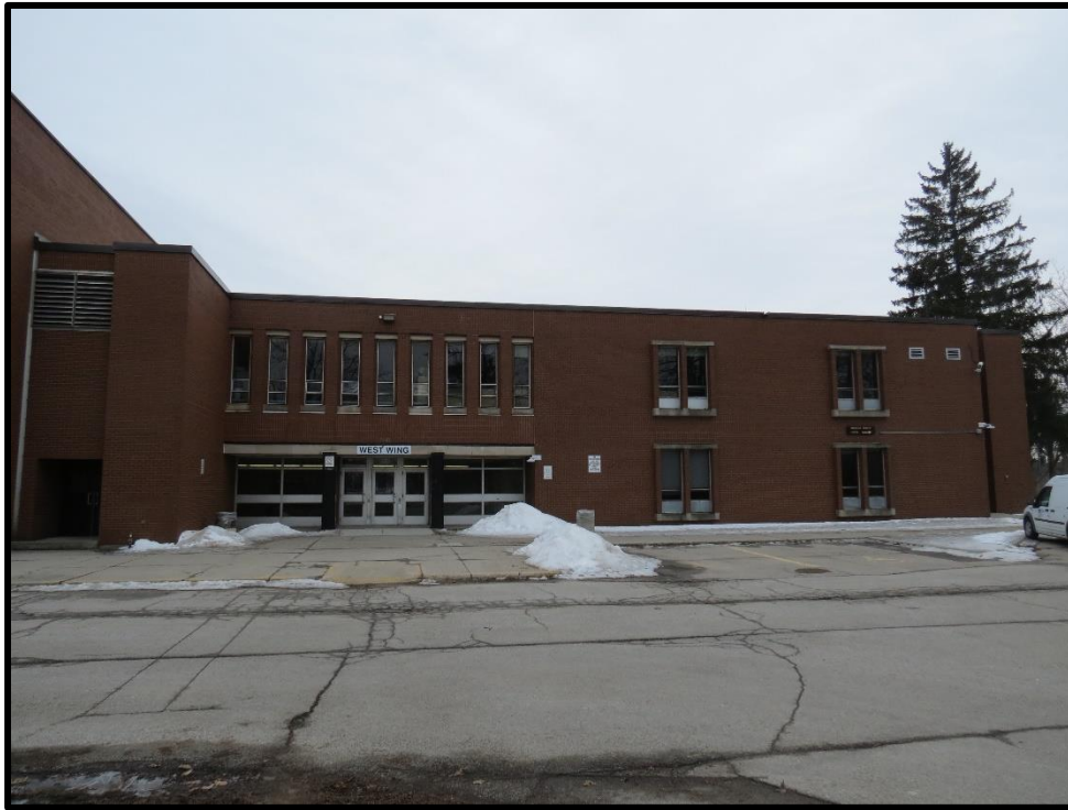
Image 12: Façade (north elevation) of West Wing (Photo taken on March 13, 2019; Facing south)
