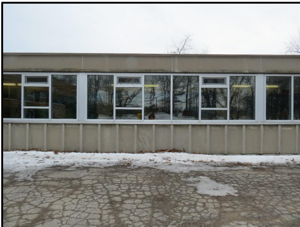
Image 11: Detail of walkway, North Elevation of West Wing (Photo taken on March 13, 2019; Facing South)
