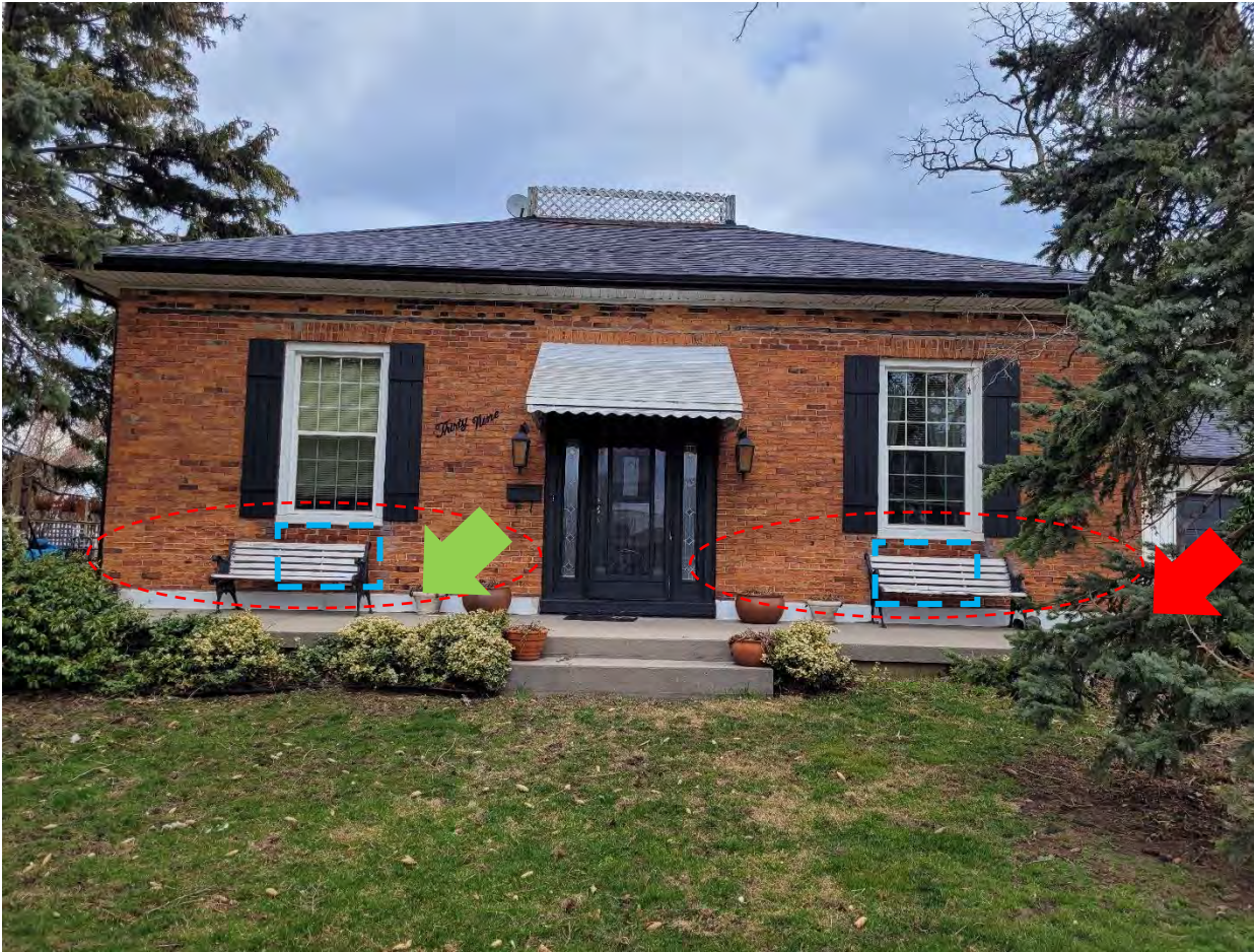
Figure 32: (Detail view of north elevation noting areas of masonry deterioration outlined in red. Evidence of conversion of French windows outlined in blue. Green arrow indicates location of Figure 21. Red arrow indicates location of Figure 22 (see below) (Source: MHBC, 2021)
