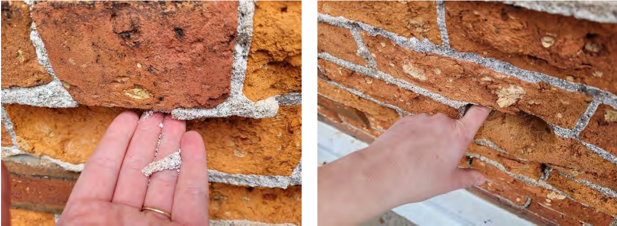
Figures 33 & 34: (left) Detail view of west elevation missing brick pillar (outlined in red), (right) Detail view of north elevation noting water damage as well as detachment between the sun room and brick pillars (Source: MHBC, 2022)
