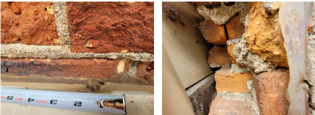
Figures 35 & 36: (left) Detail view of north elevation caulking noting areas where water is able to penetrate, (right) Detail view of south-east corner of the building where bricks are missing and crumbling above the foundation, (Source: MHBC, 2022)
