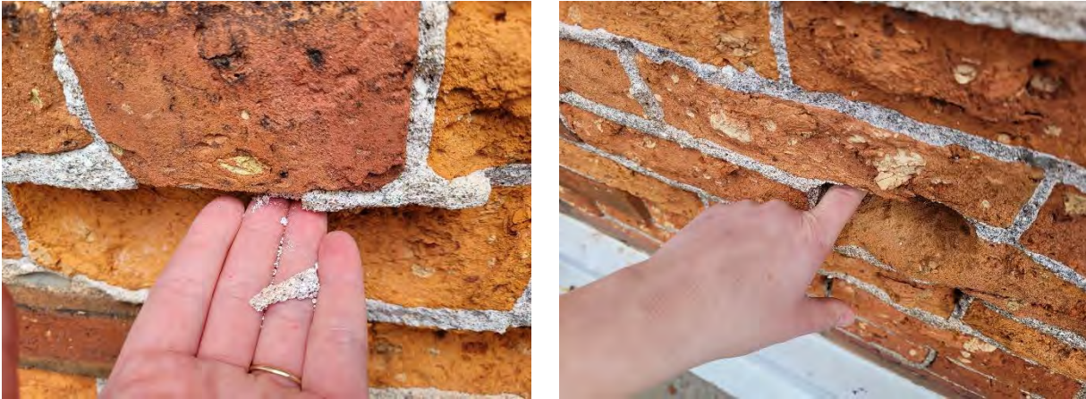
Figures 33 & 34: (left) Detail view of west elevation missing brick pillar (outlined in red), (right) Detail view of north elevation noting water damage as well as detachment between the sun room and brick pillars (Source: MHBC, 2022)
