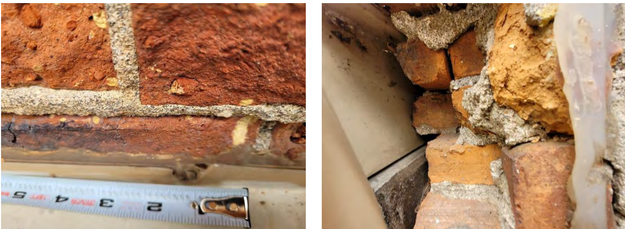
Figures 35 & 36: (left) Detail view of north elevation caulking noting areas where water is able to penetrate, (right) Detail view of south-east corner of the building where bricks are missing and crumbling above the foundation, (Source: MHBC, 2022)
