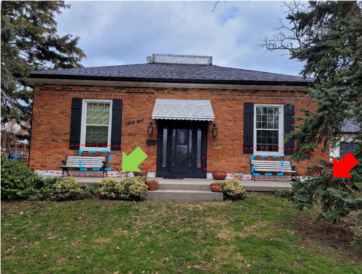
Figure 32: (Detail view of north elevation noting areas of masonry deterioration outlined in red. Evidence of conversion of French windows outlined in blue. Green arrow indicates location of Figure 21. Red arrow indicates location of Figure 22 (see below) (Source: MHBC, 2021)
